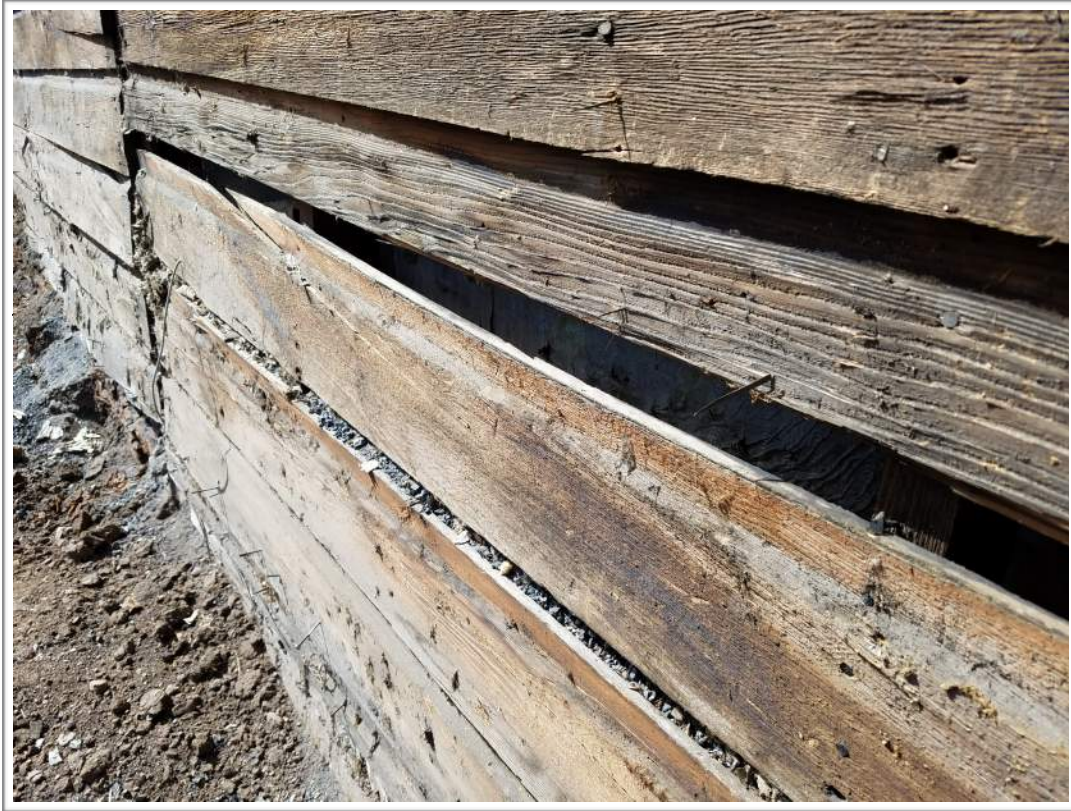
Photo #25 East Facade Siding Condition
