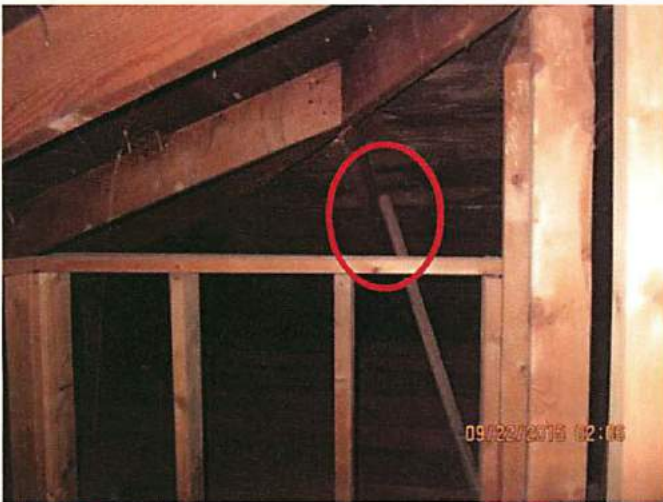
Photo 5 Support member not properly fastened
