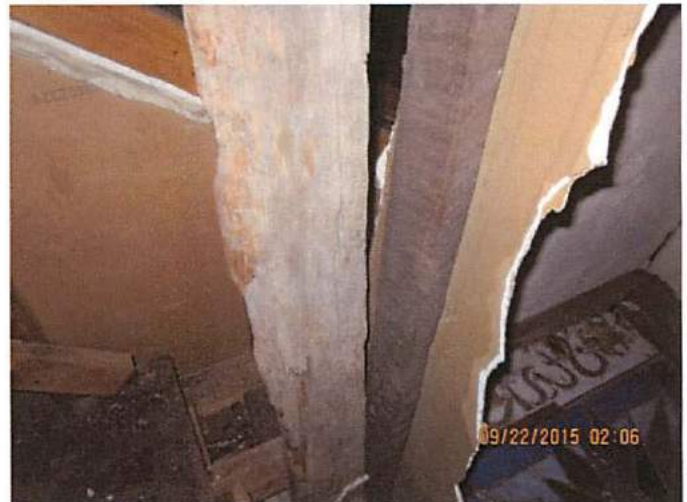
Photo 4 Structural members not properly supported
