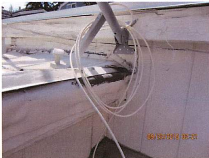
Photo 30 Possible location of water infiltration
