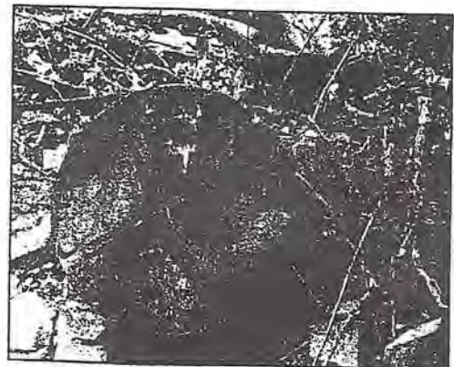
Figure 35 – Lower drum of boiler.
