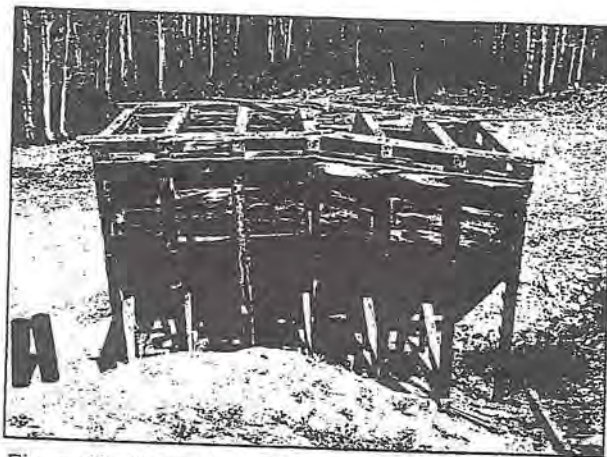
Figure 43 – Rear view, showing sagging corner.
