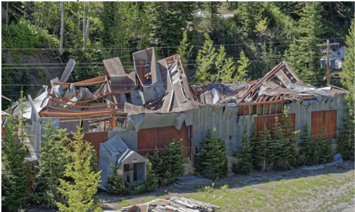
Figure 5: Image showing snow damage in the Spring 2024
