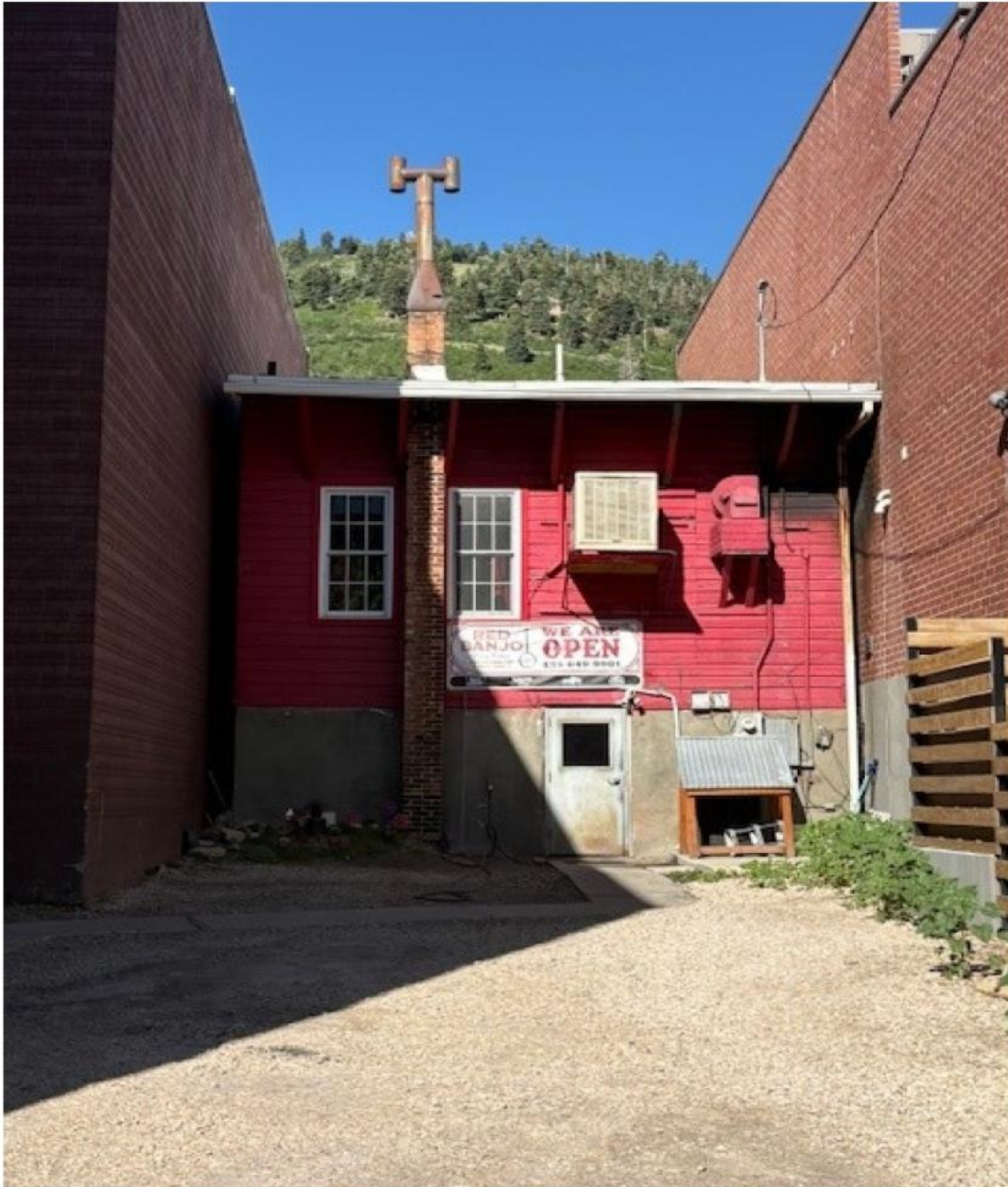
Figure 9: Applicant's photo submittal showing the rear façade, with most materials replaced in 1976. The Applicant's Historic Preservation Plan indicates the brick of the chimney is historic but is proposed to be removed.
