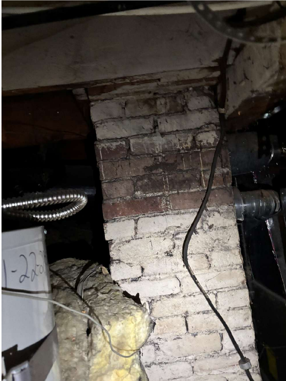
Figure 8. The southernmost, interior chimney extends through the basement and may have originally connected to a stove in the kitchen. It is no longer apparent in the kitchen.
