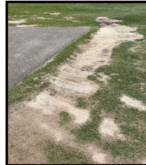
Uneven Cart Path Transition to Turf
