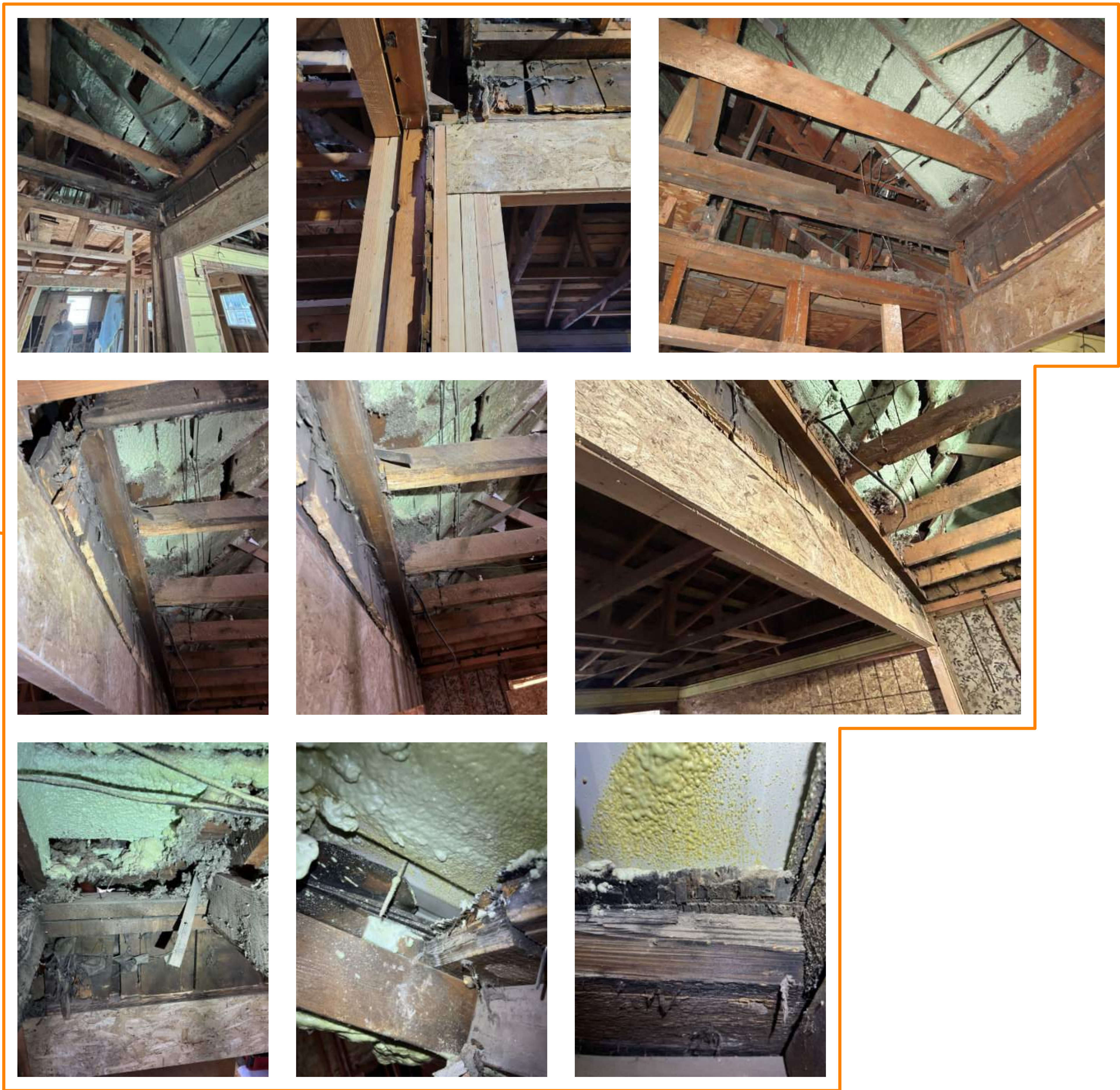
Advanced rotting paired with improper framing
