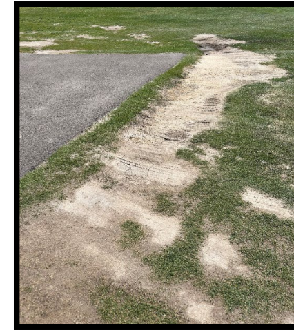
Uneven Cart Path Transition to Turf
