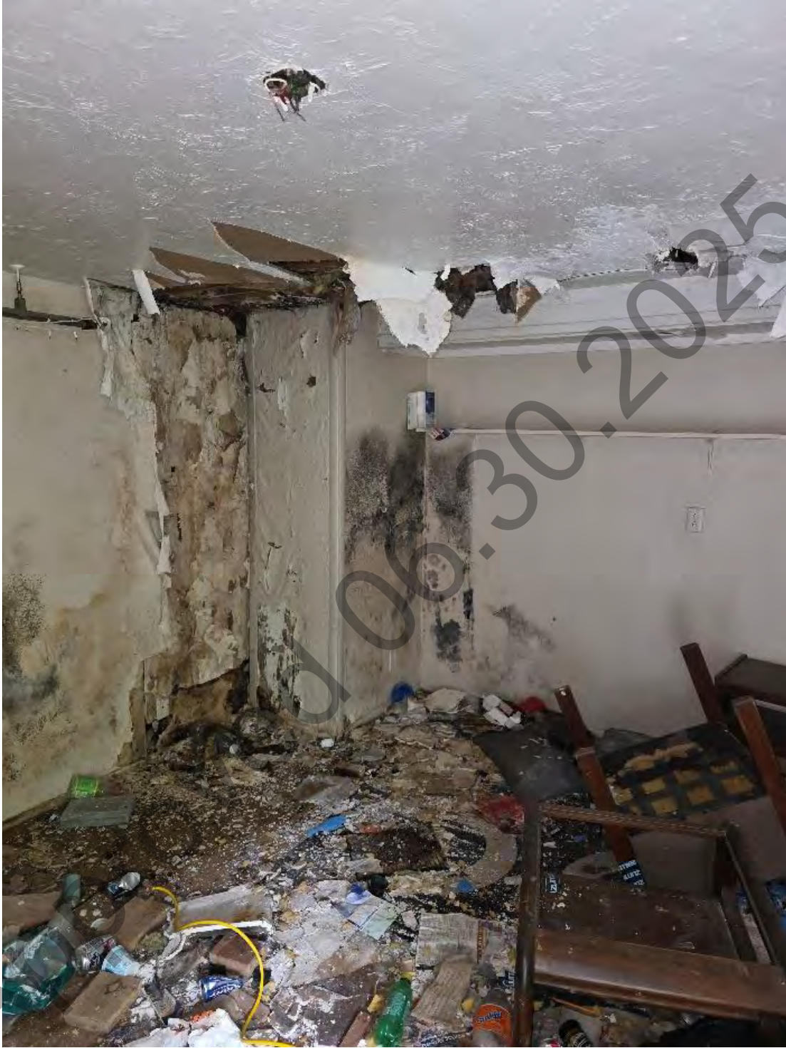
South Basement Apartment Living Room – Three (3) dead raccoons, feces, visible mold on all walls within the basement area.
