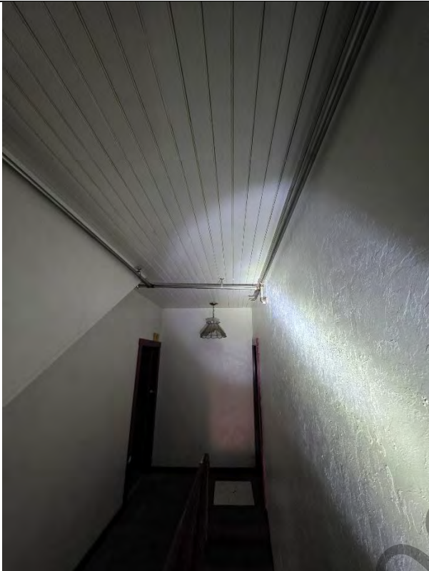
Green wood ceiling positive for lead
