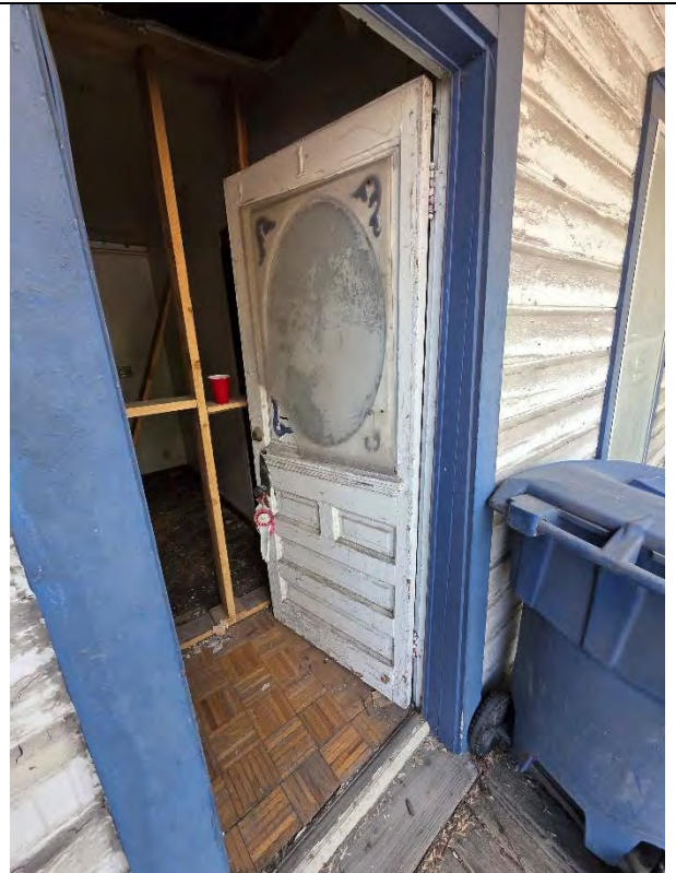
Lead exterior door, siding and door frame
