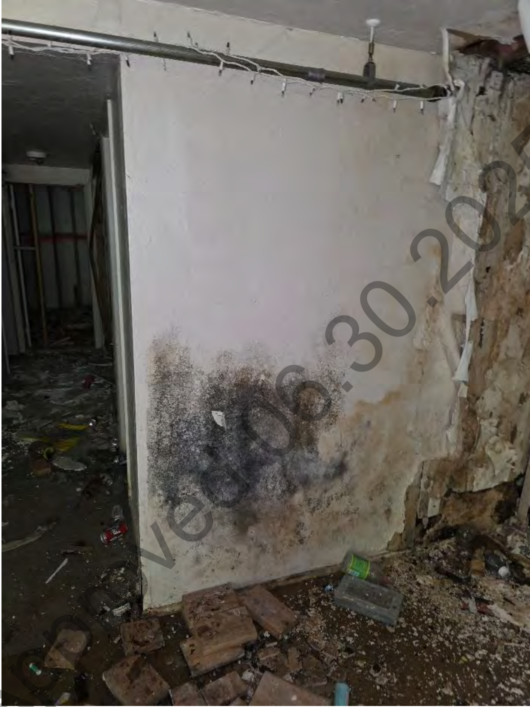
Visible mold growth on wood paneling Office 103/104.
