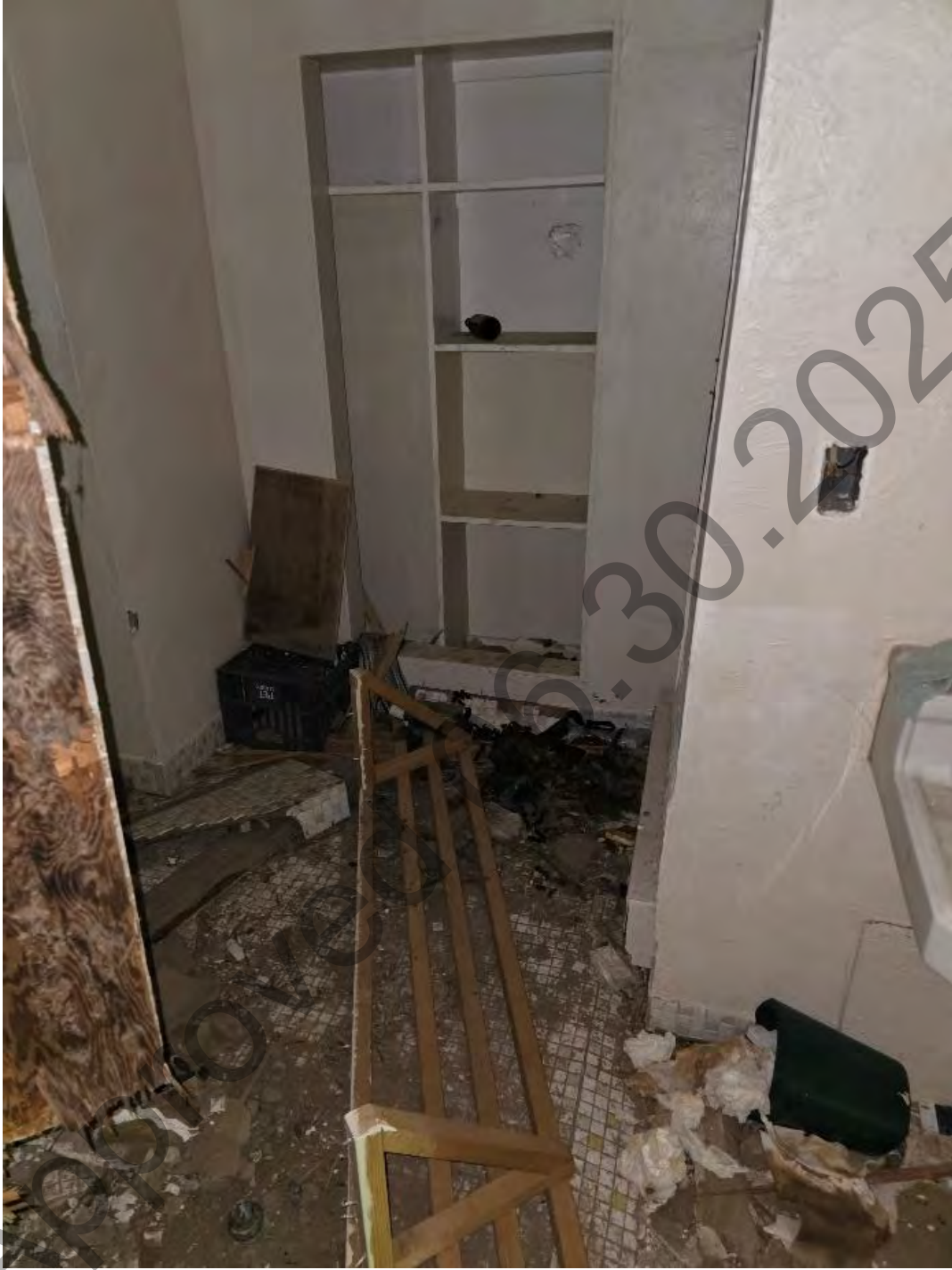
Visible mold growth on sheetrock wall Basement South Apartment Bathroom.
