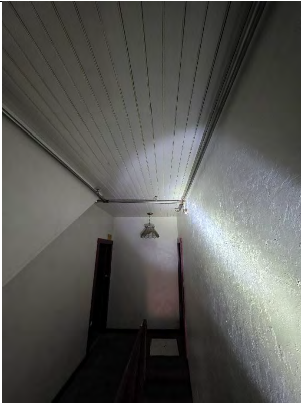
Green wood ceiling positive for lead
