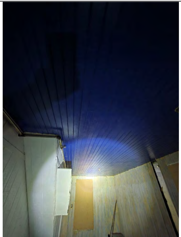
Blue wood ceiling positive for lead
