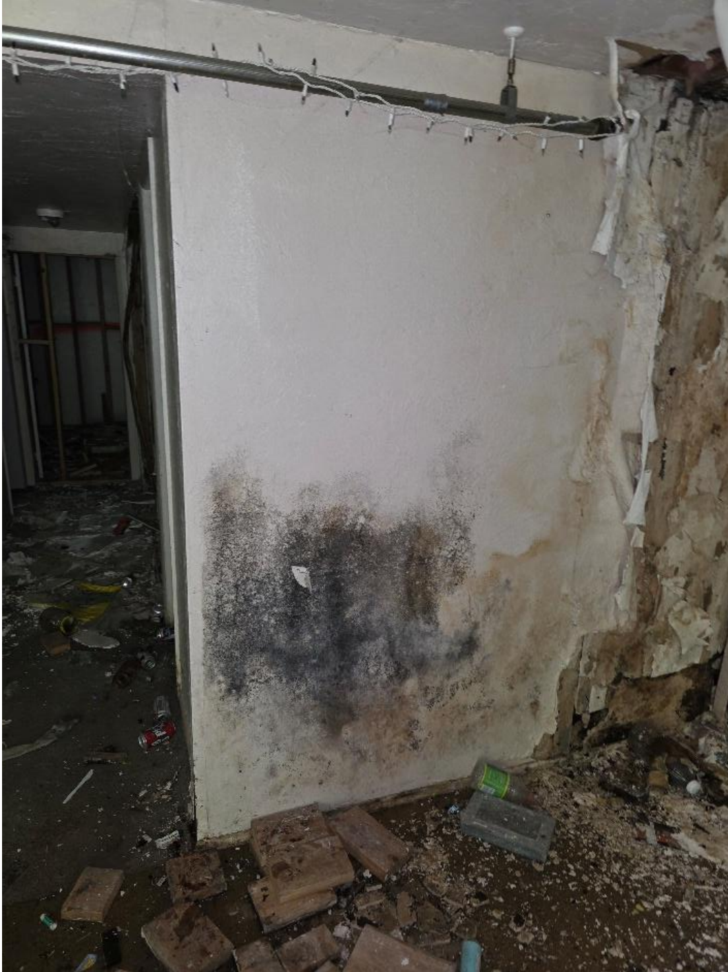
Visible mold growth on wood paneling Office 103/104.
