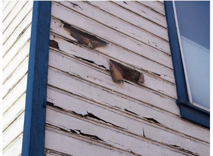
Example of Peeling paint on West Facade
