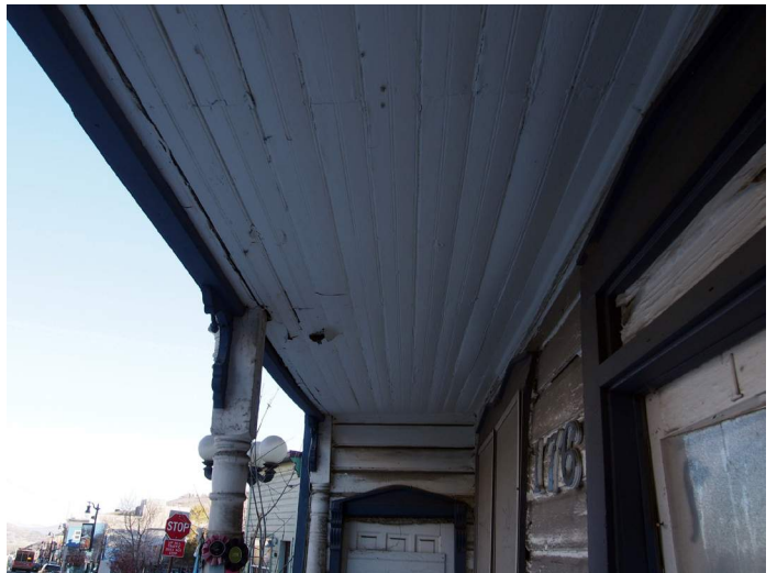
Front Deck soffit bowing
