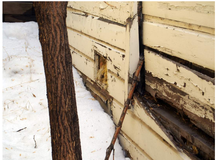
South facade trim issues
