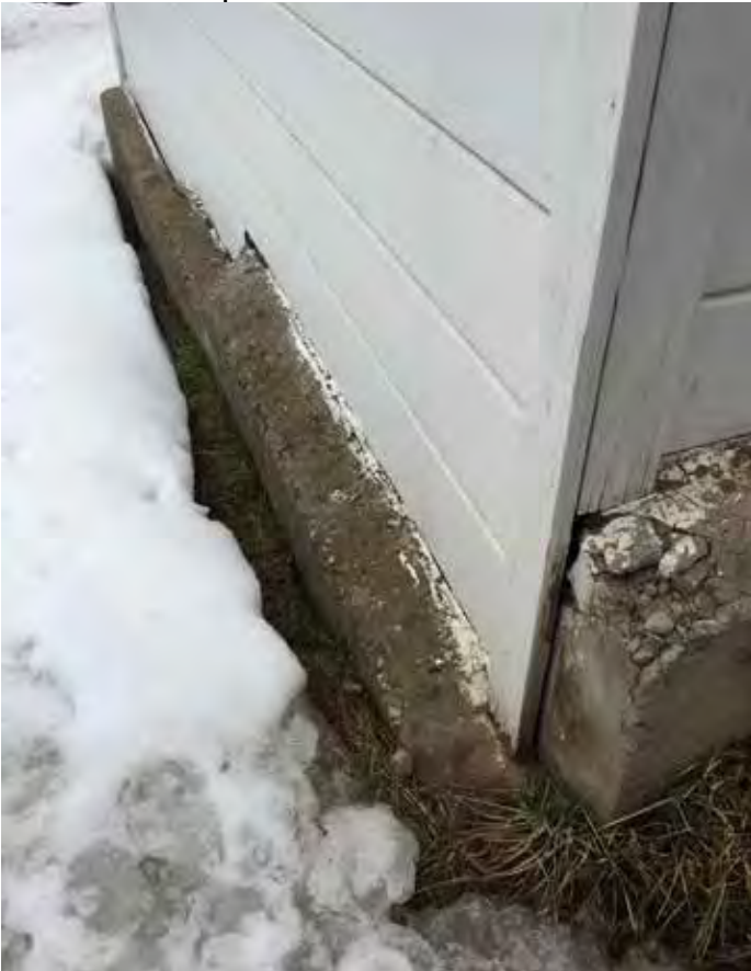
Photo #35: Exposed Foundation At Addition
