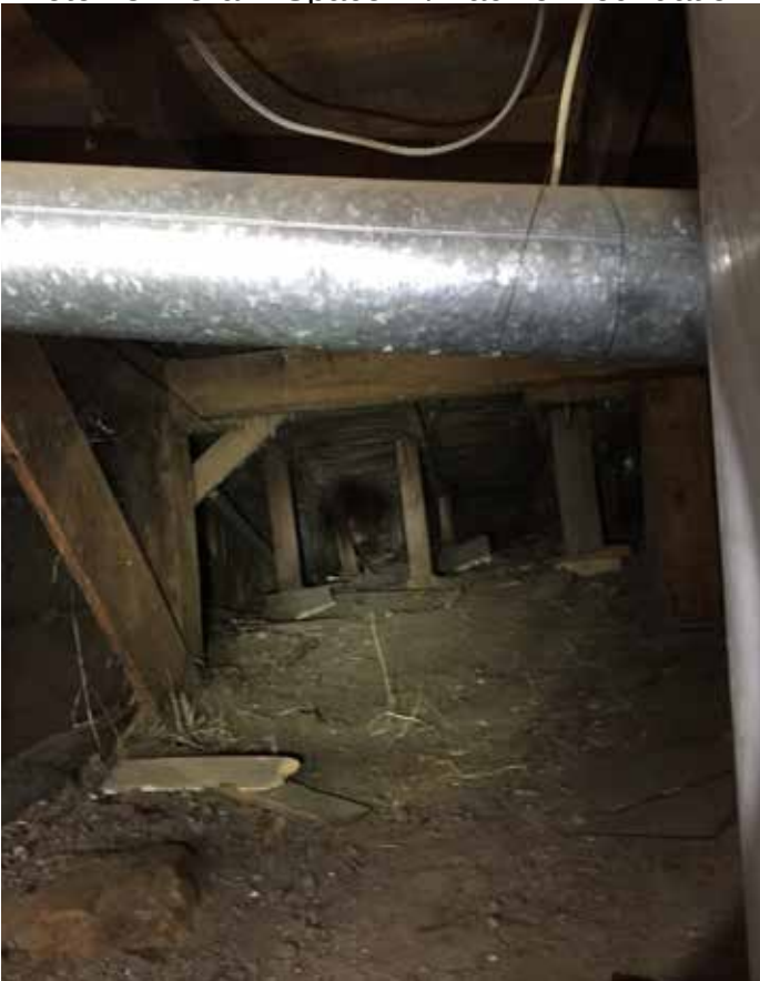
Photo #37: Crawl Space W/ Lack of Foundation
