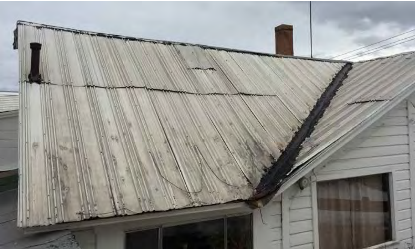
Photo #18: View of Overbuilt Roof Above Kitchen
