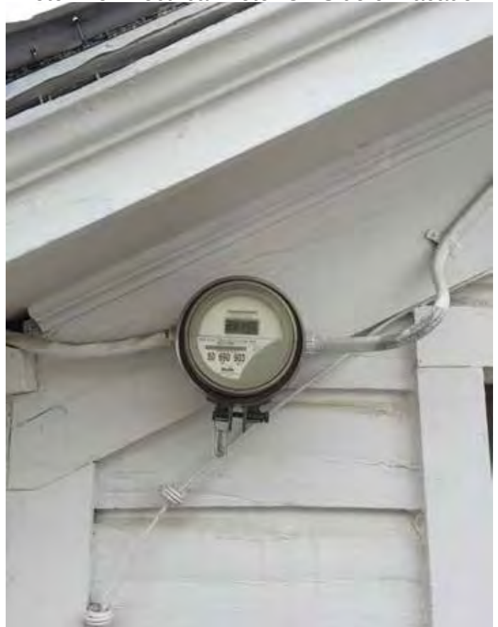
Photo #45: Electrical Meter On Side of Facade
