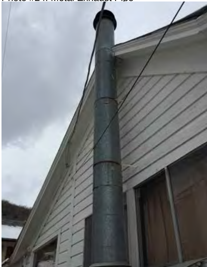
Photo #24: Metal Exhaust Pipe
