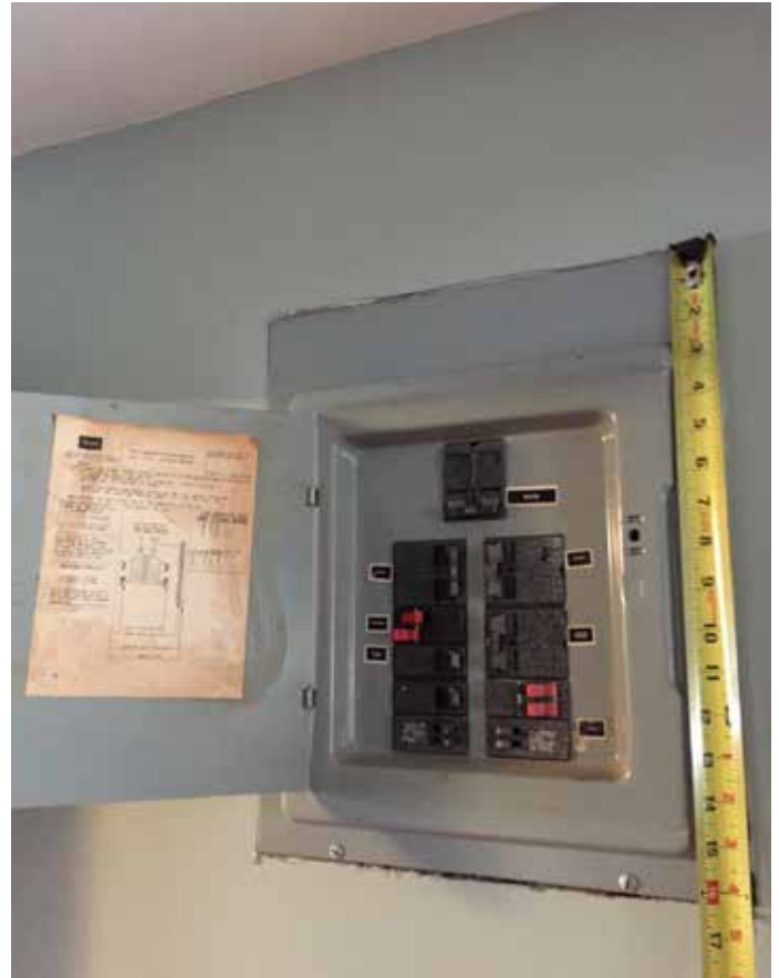
Photo #47: Electrical Panel In Kitchen
