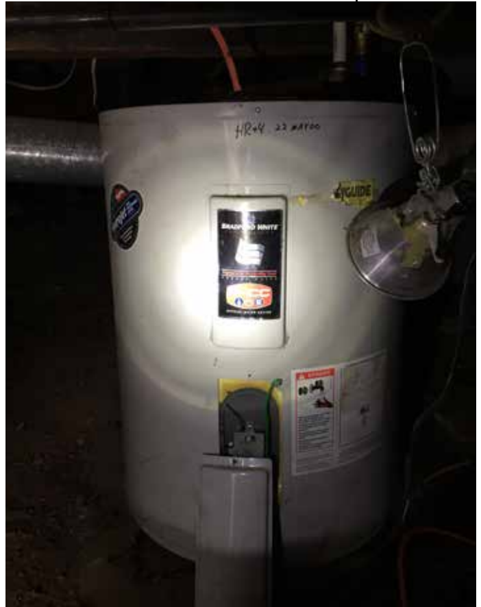
Photo #43: Water Heater In Crawl Space
