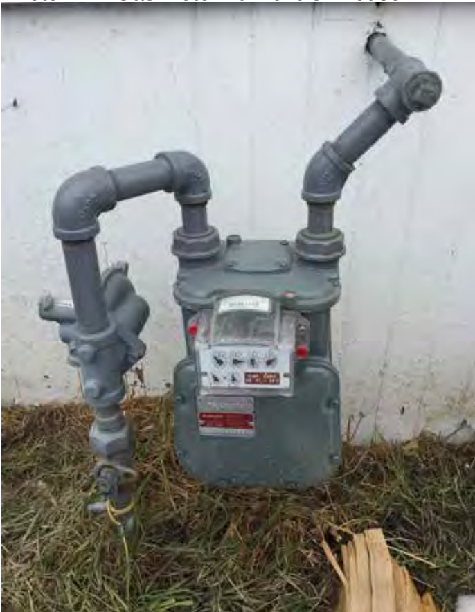
Photo #44: Gas Meter At Front Of House
