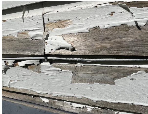
Figure 5: Close-up view of peeling siding
