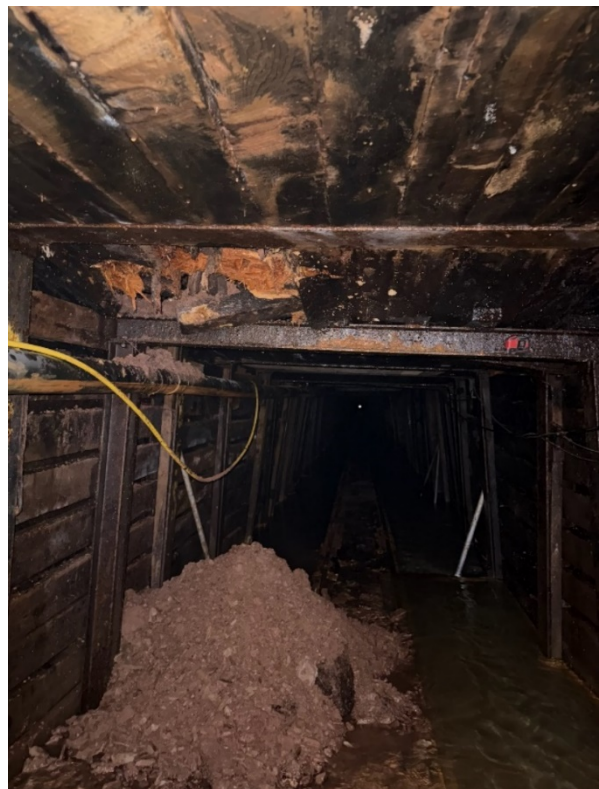
Figure 1: Tunnel condition and small collapse in Oct.24
