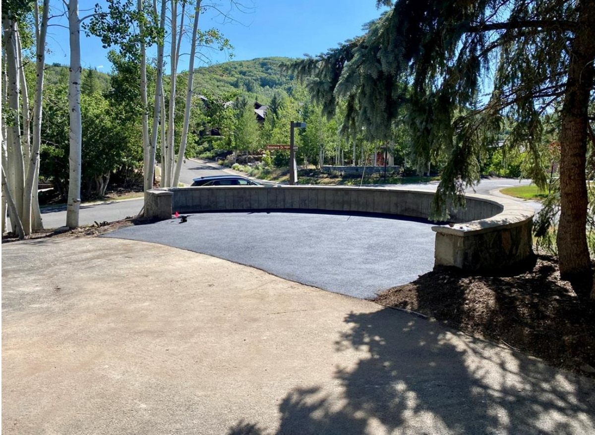
Figure 5: Completed Construction at 3295 Thistle Street in violation of LMC § 15-2.13-3 and § 15-3-3(H)(1) and without a Building Permit
