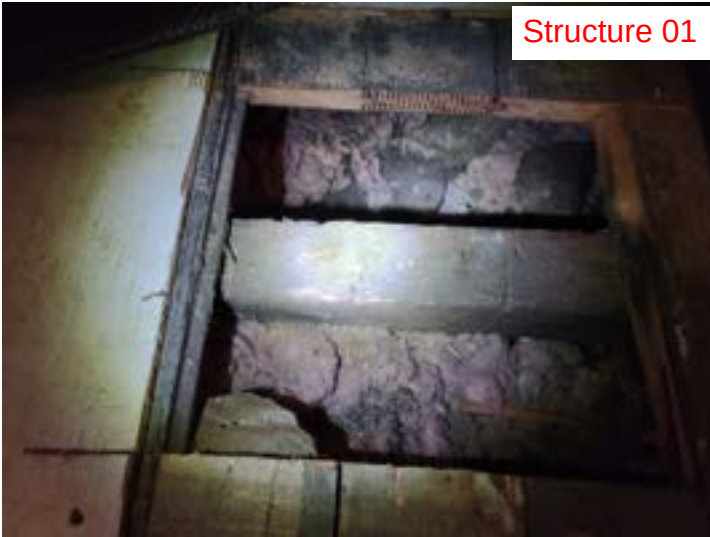
Exposed floor joists sitting on earth at front historic portion of house.
