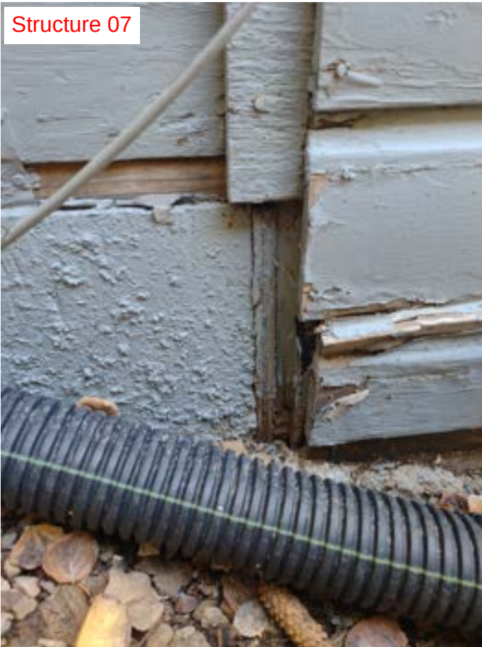
Transition between foundation at 1988 addition, and rim joist sitting on grade at historic portion of house.
