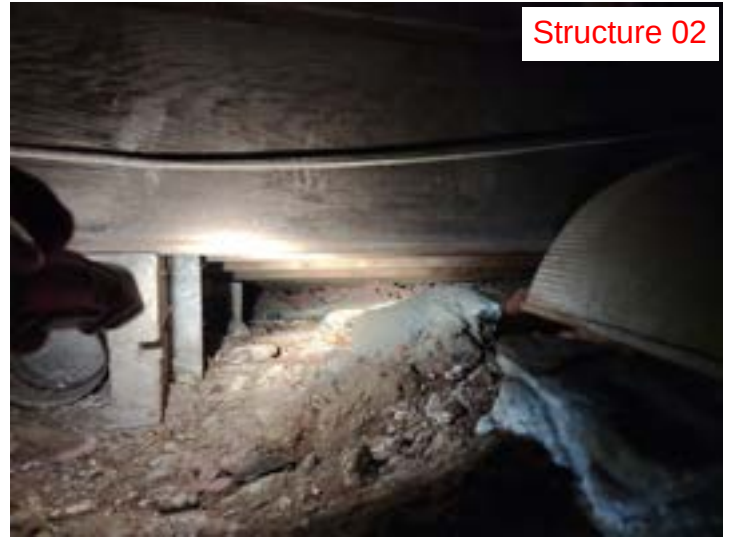
Floor joists sitting on CMU blocks and earth at front historic portion of house.
