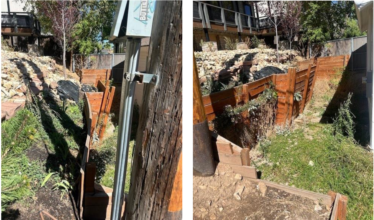
Figures 1 and 2: Applicant's photos showing existing failing wood retaining wall at 501 Park Avenue.
