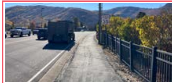
Kearns Blvd Sidepath | Deficient
