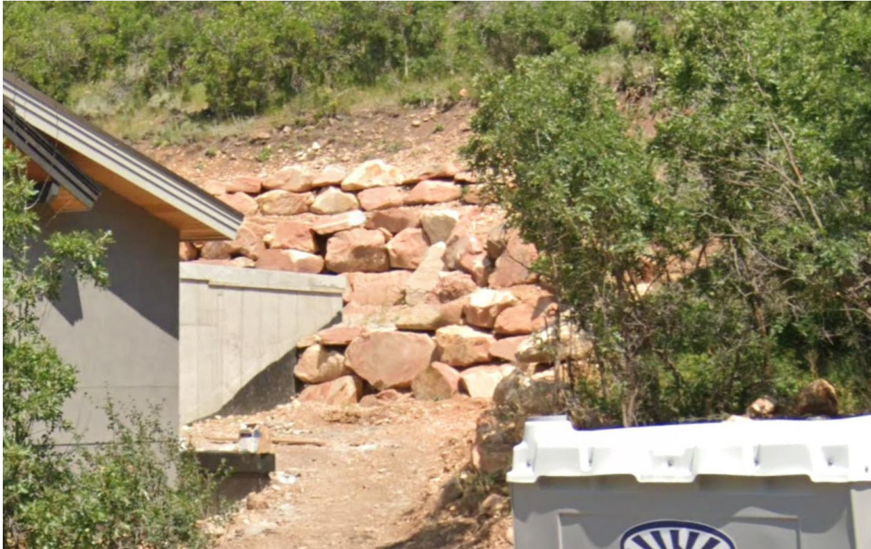
Figure 1: Google Maps screenshot showing retaining walls in the rear of the SFD at 950 Aerie Drive in July 2024.
