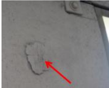
Figure 1: Failing concrete patch
