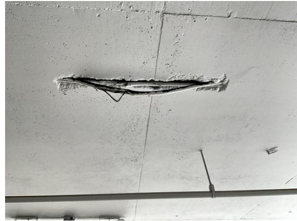
Figure 19: Damaged PT Tendon
