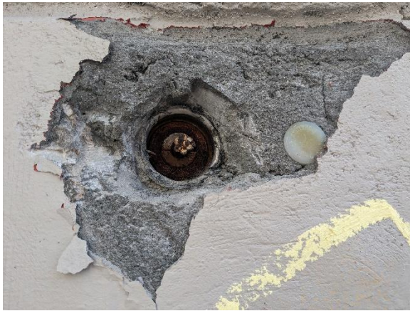
Figure 18: Exposed Grout Pocket at De-Stressed Tendon
