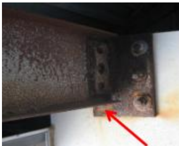
Figure 9: Structural steel rust & scaling
