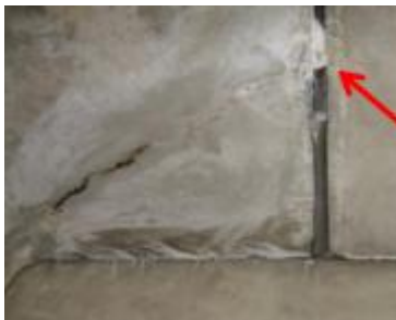
Figure 7: Leaking and leaching concrete
