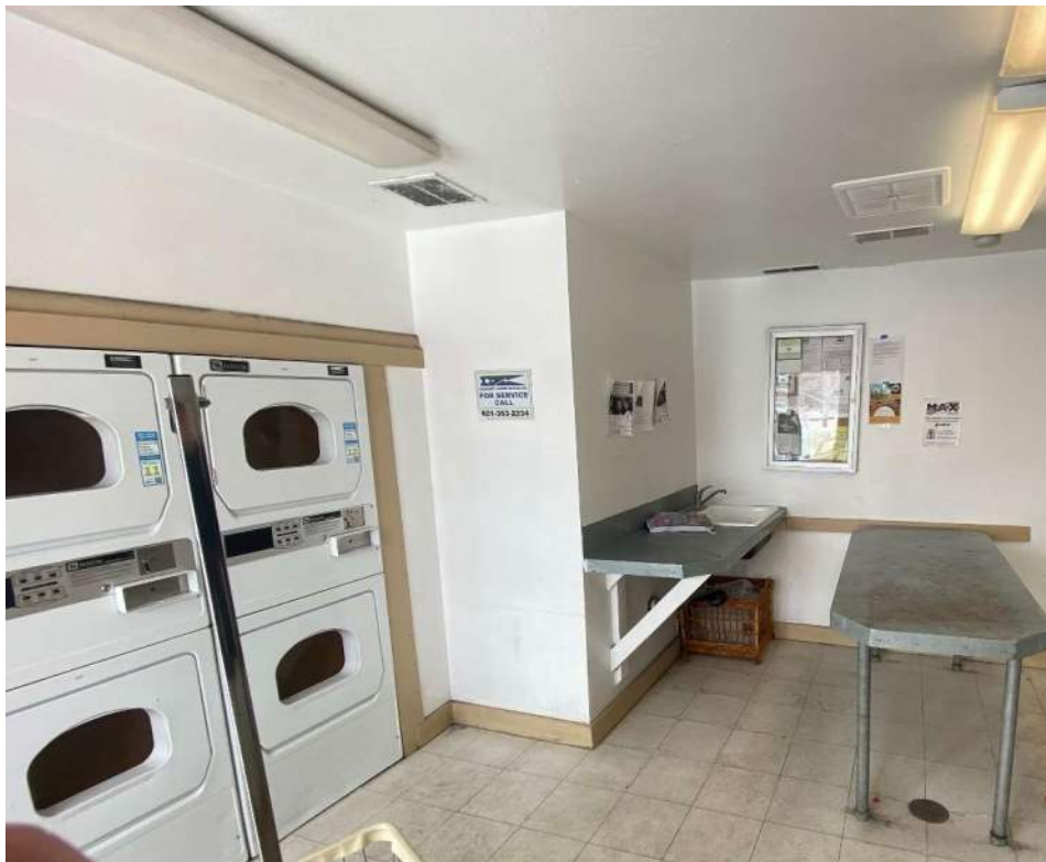
Photo 12. Parkside Apartments: Laundry facility.
