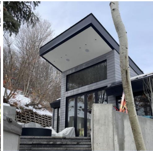
Existing, unapproved roof.
