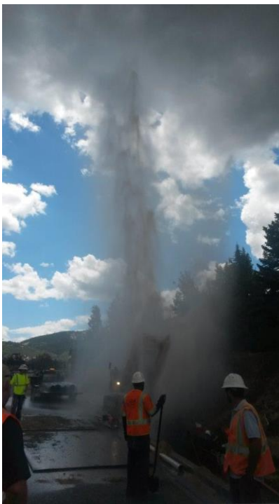
Figure 1 Leaky Pipe that Failed on 224
