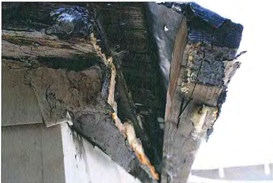
7. Fascia at southeast corner
