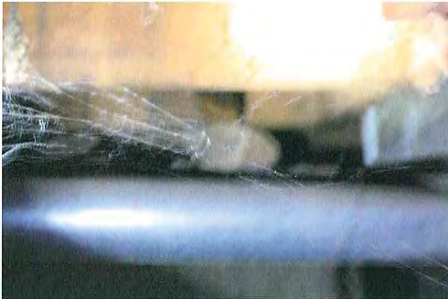
Duct work-exposed no insulation
