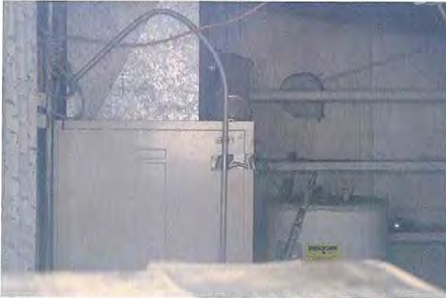
1.Mechanical room-furnace and water heater
