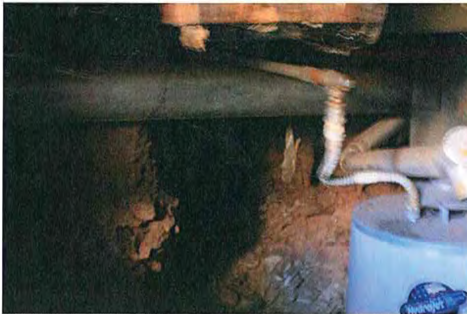
Hot water heater-venting?
