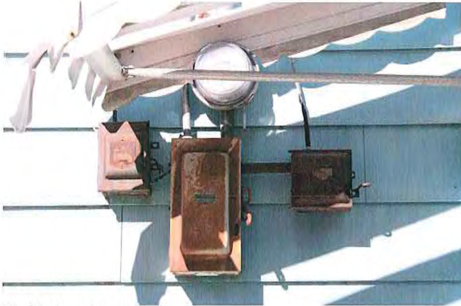
Electrical service-south elevation
