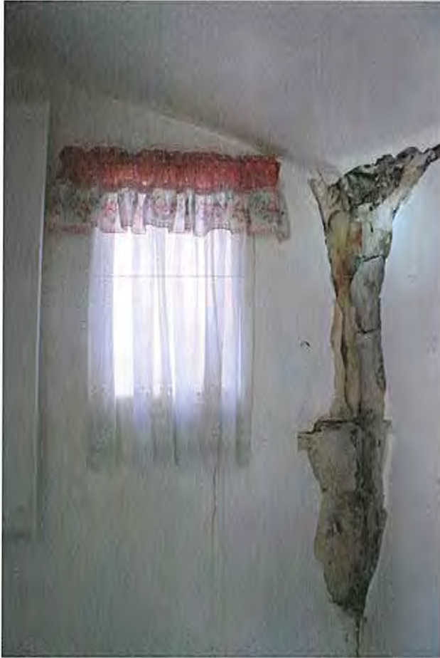
Visible mold-probably hidden mold
