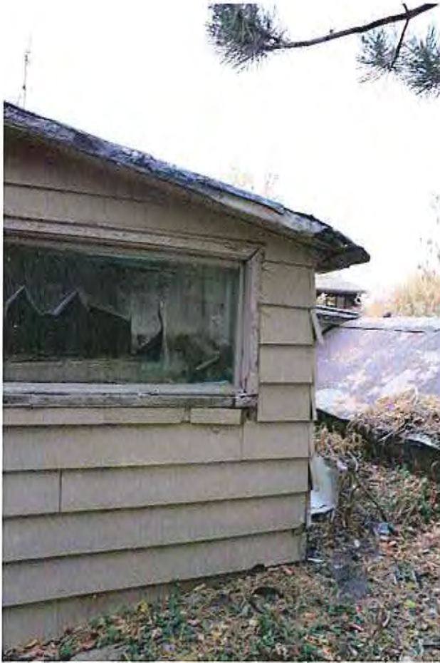
5. Southeast corner mechanical room
