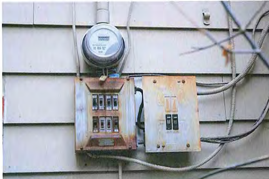
2. Closeup electrical service
