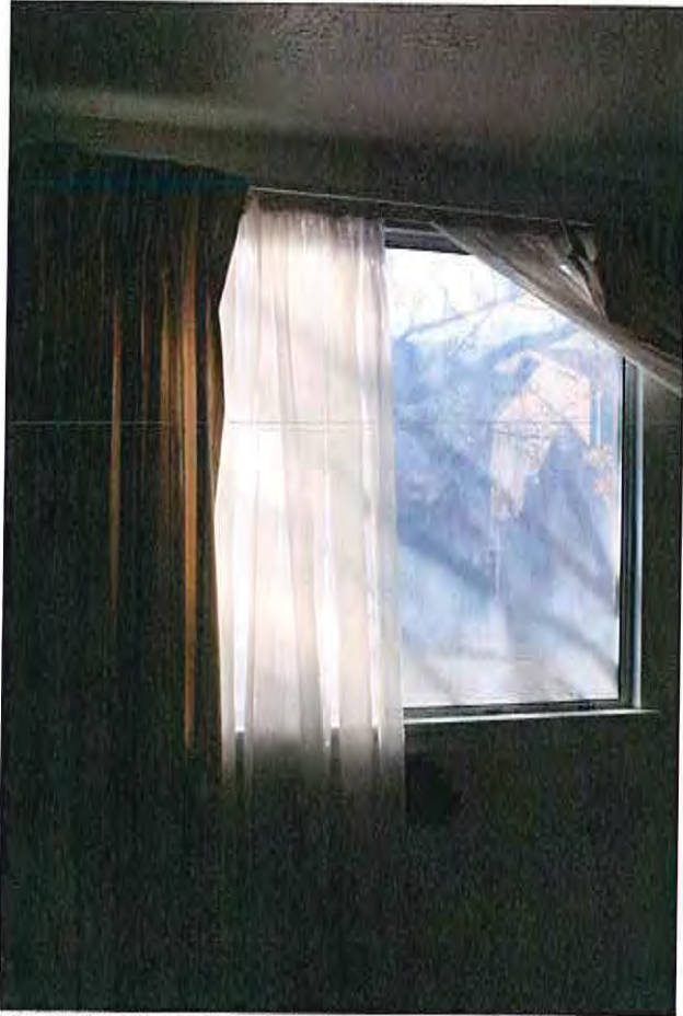
Front-west window interior-casing modified
