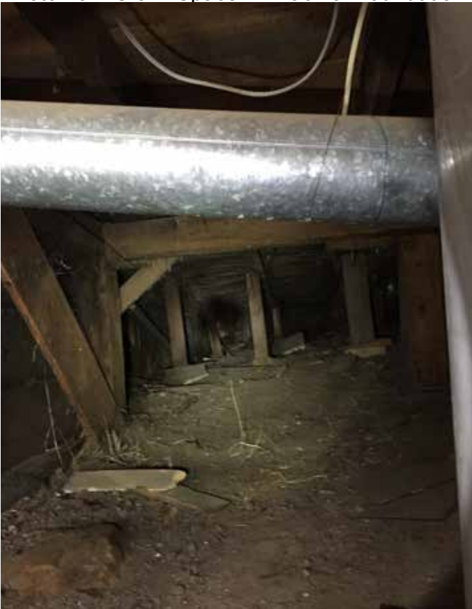
Photo #37: Crawl Space W/ Lack of Foundation
