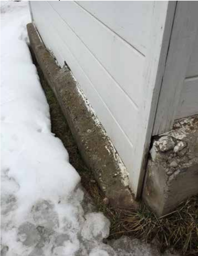
Photo #35: Exposed Foundation At Addition
