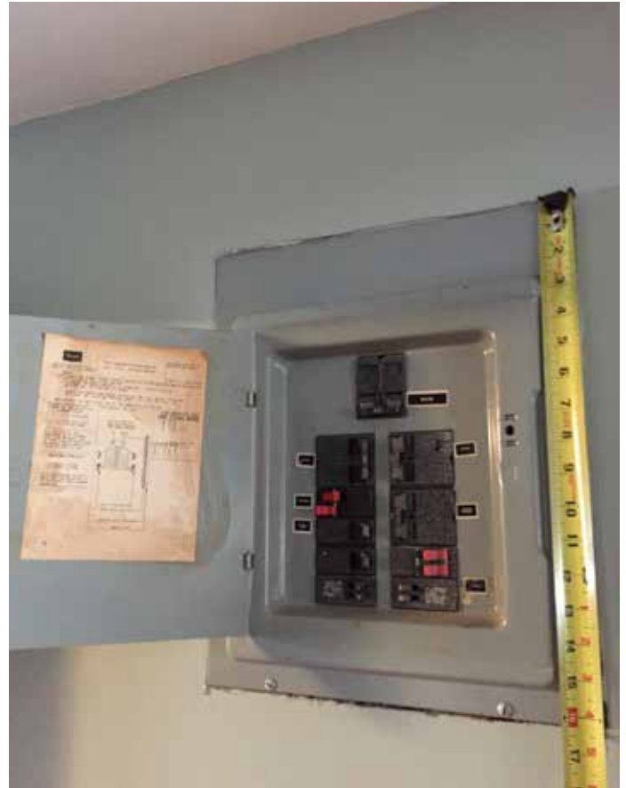
Photo #47: Electrical Panel In Kitchen
