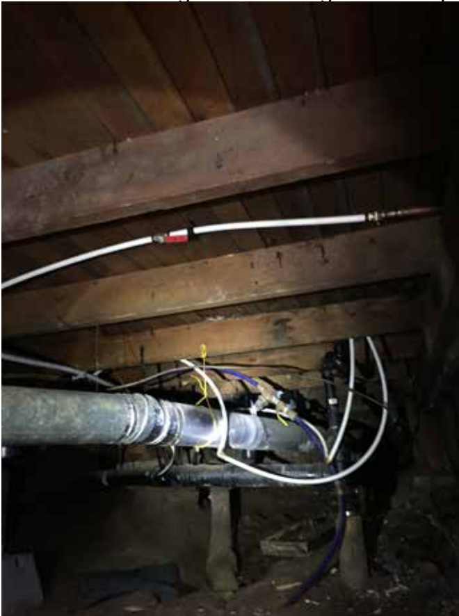
Photo #46: Ducting and Plumbing in Crawl Space
