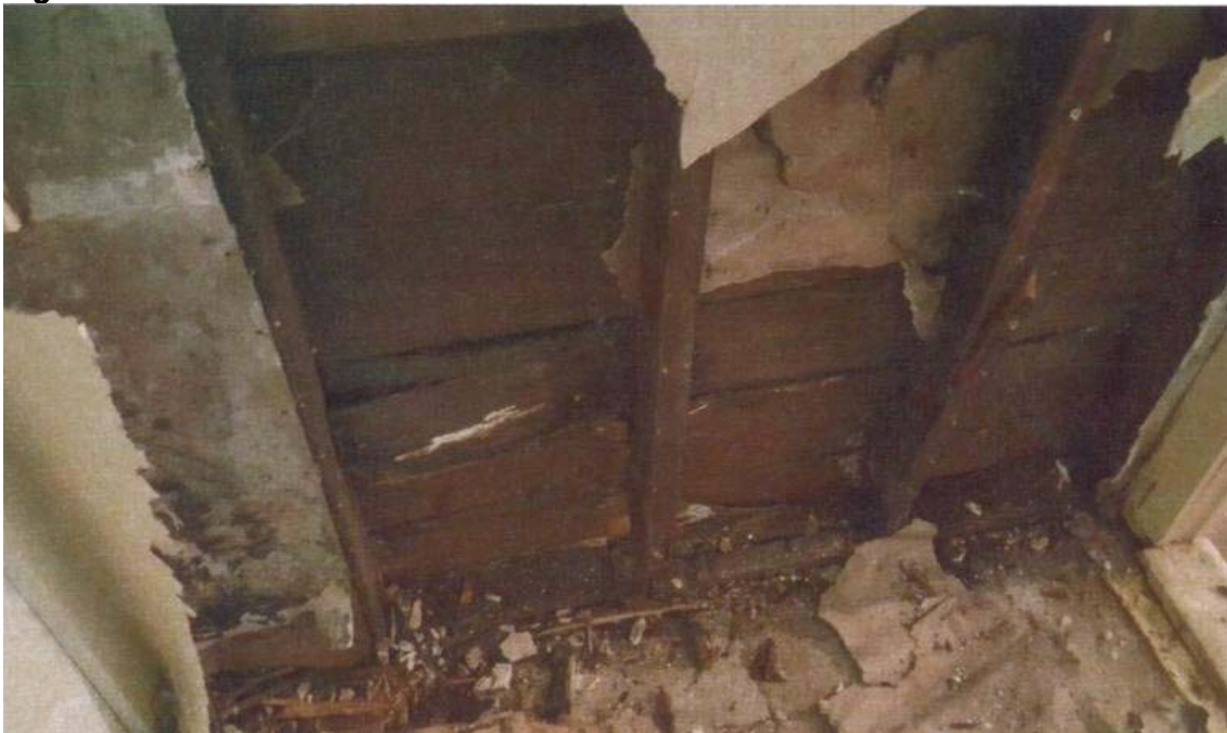
Rotted wall in the bathroom.
