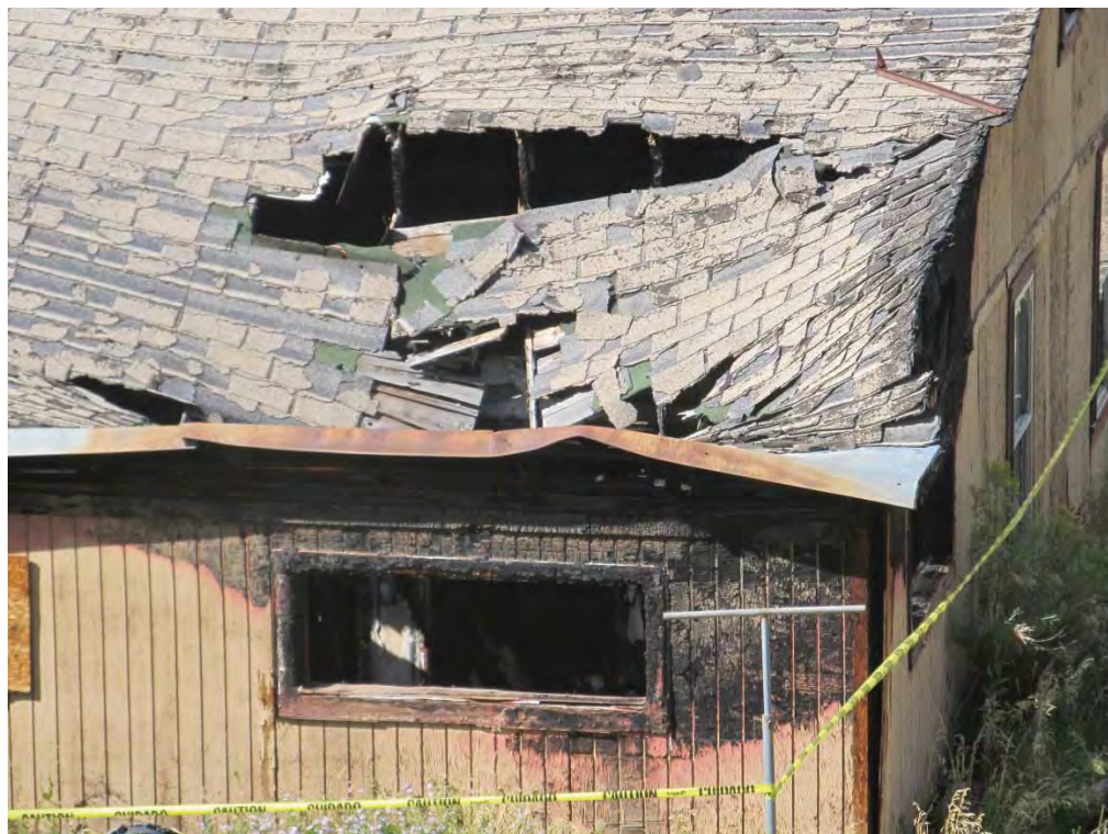
Fire Damage on South Elevation
