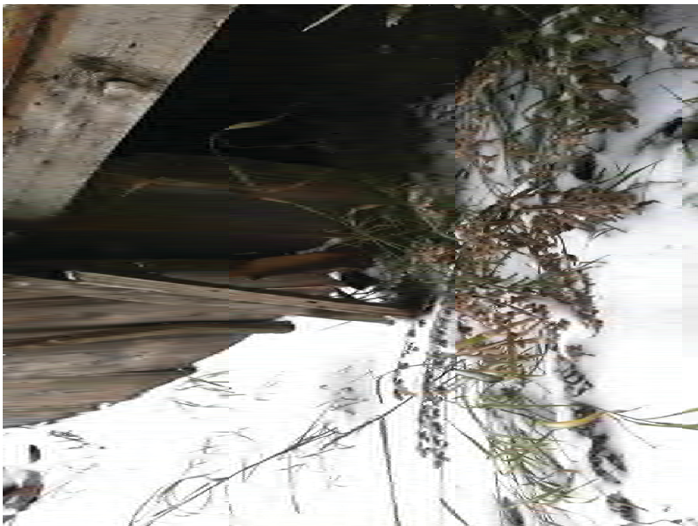
Dilapidated vertical wood siding used on porch (as seen in 1930s tax photo)
