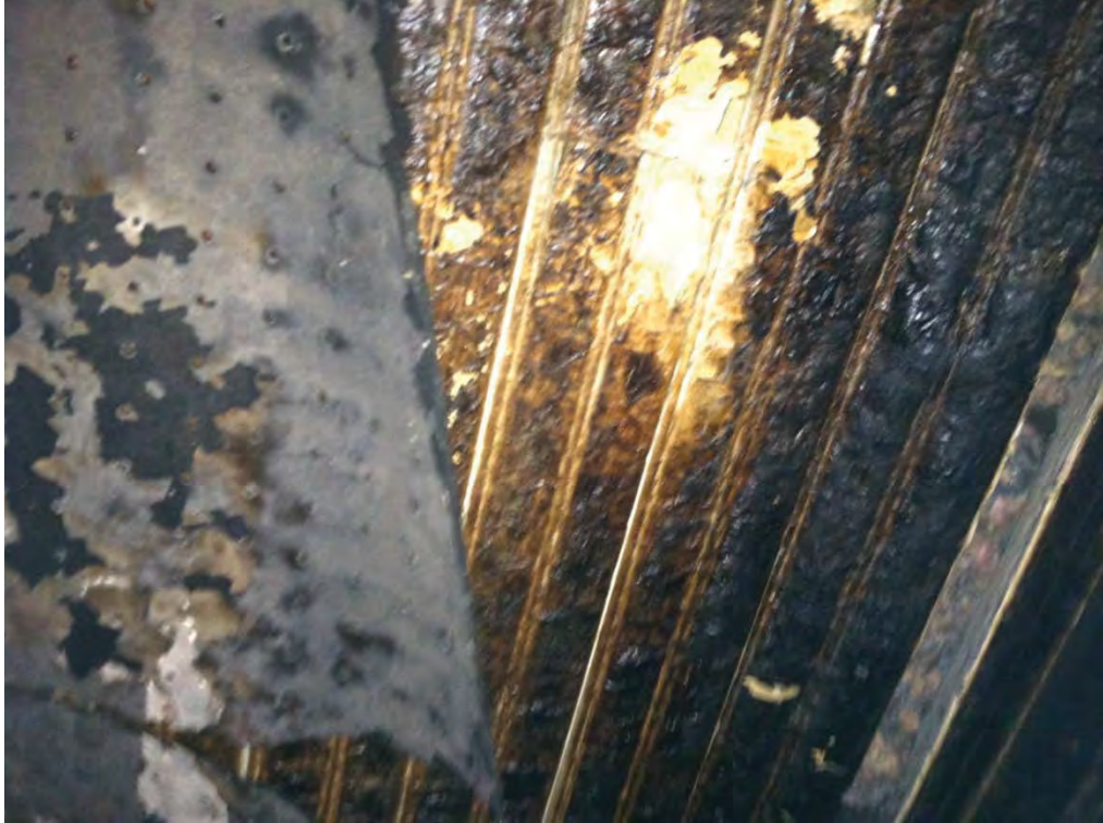
Charred bead-board ceiling in kitchen
