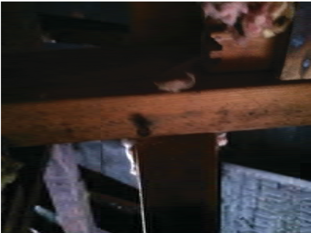
Antique nail and charred roof structure, interior
