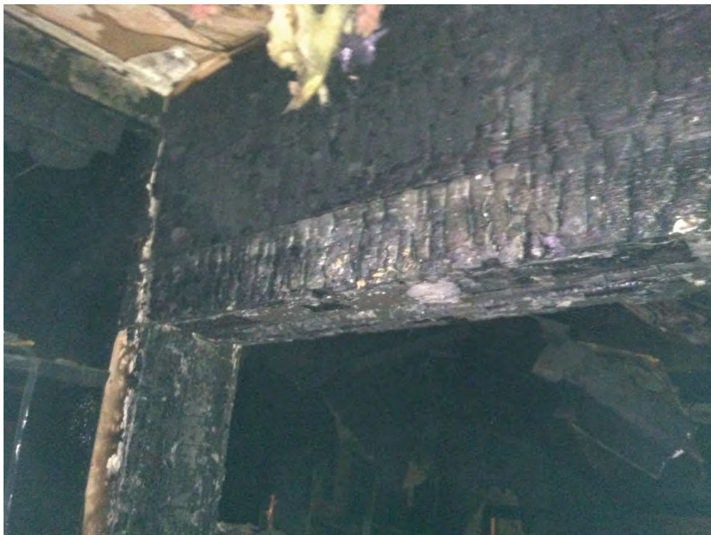
Charred ceiling structure, interior
