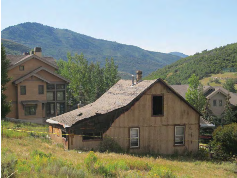
East Elevation (note fire damage)
