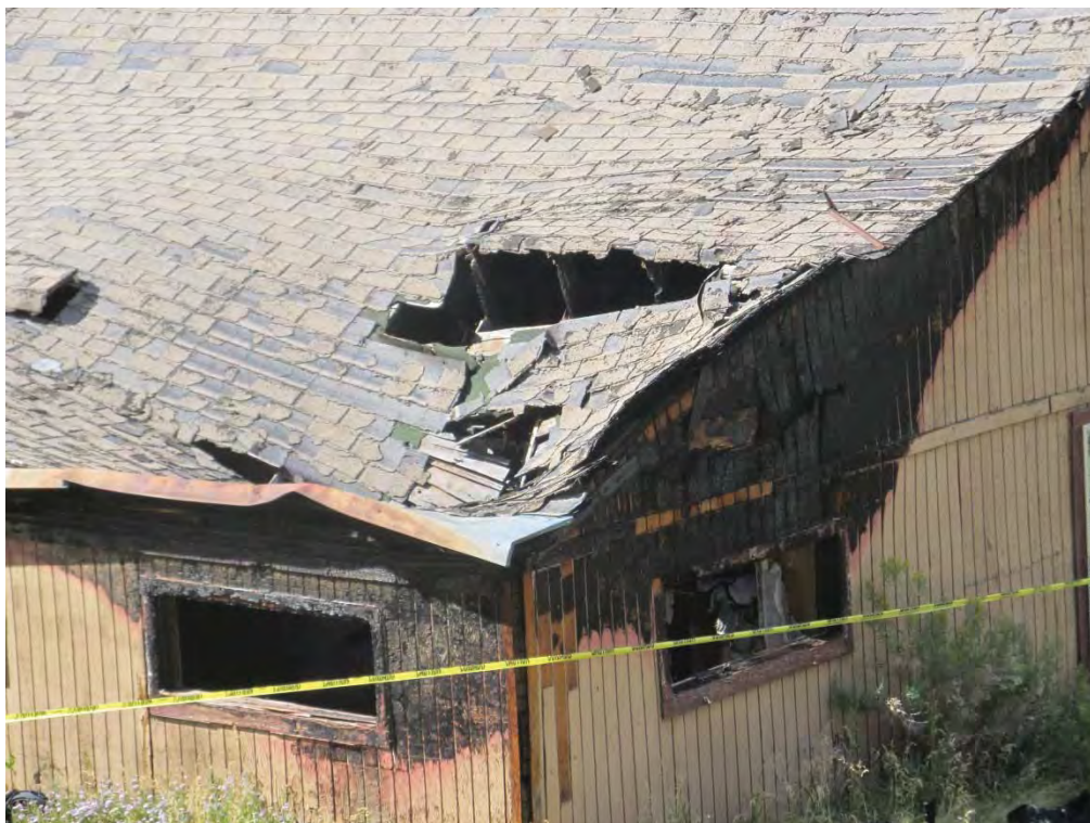
Fire damage at southeast corner
