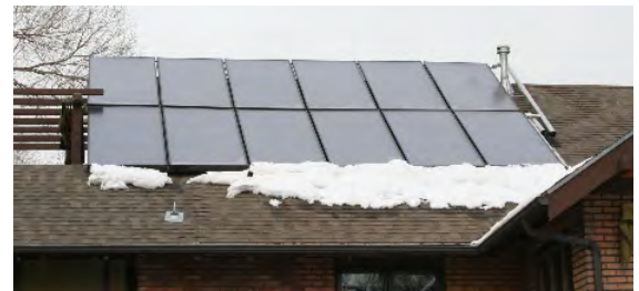
Solar panels visual impacts are minimized
