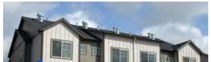
Mechanical vents reflect architectural style
