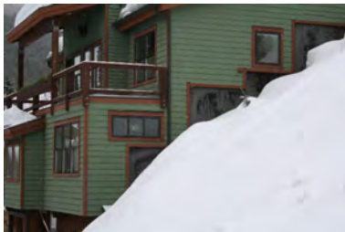
Foundation wall too exposed
