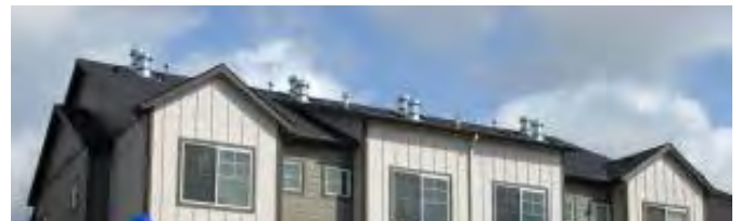
Mechanical vents reflect architectural style
