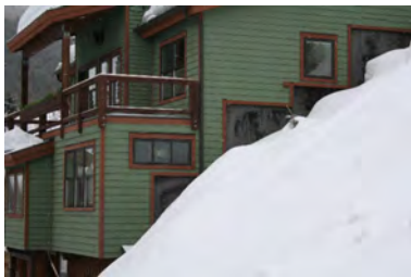
Foundation wall too exposed
