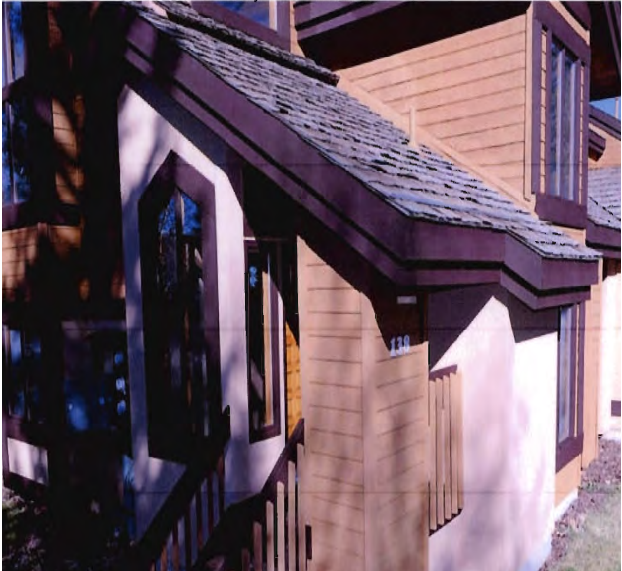
Side-entry unit as constructed
