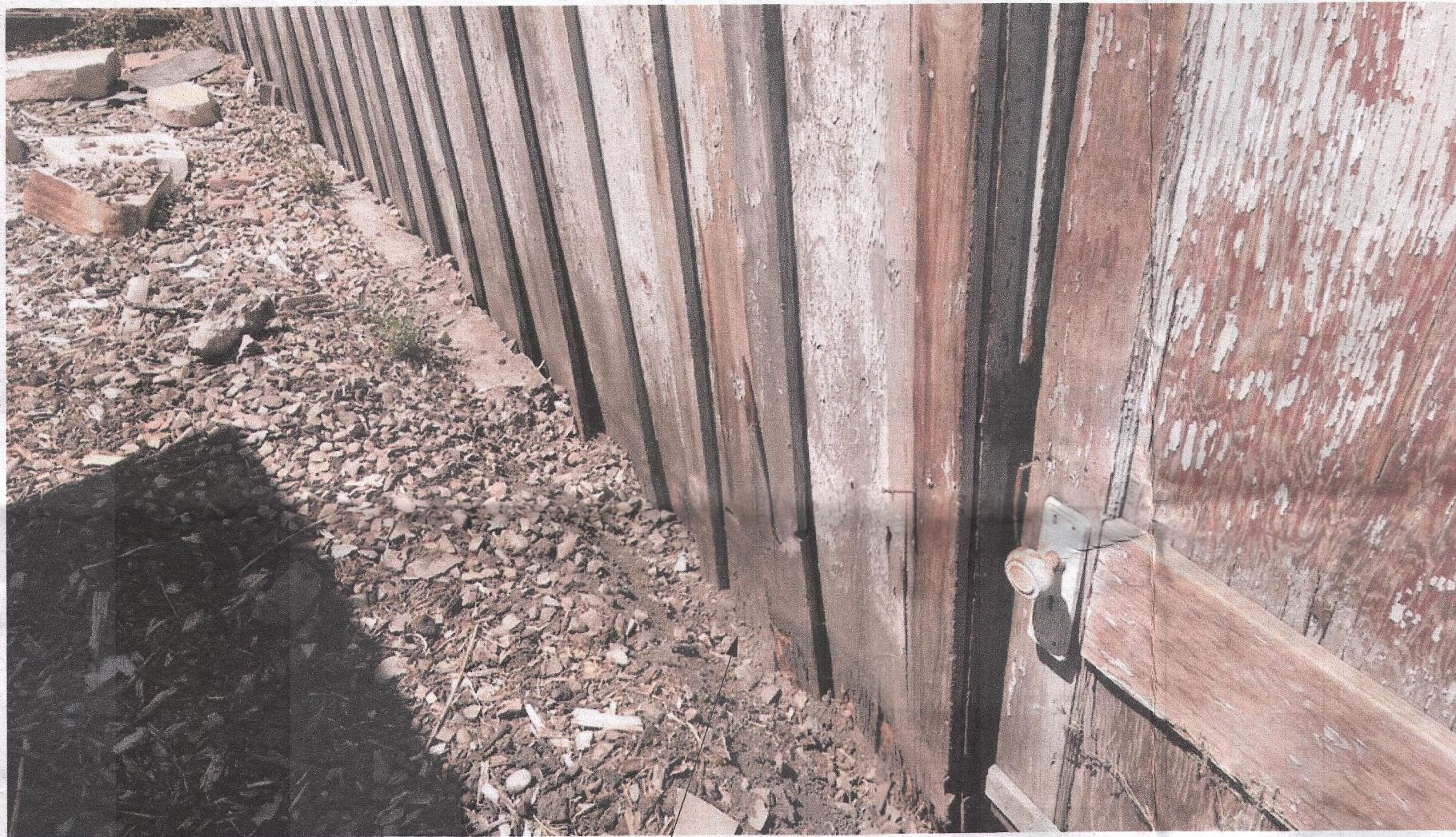
Soil Has been Built Up Over Years Impacting Integrity of Board & Batten - Salvage & Panelize Walls - Incorporate All Useable Materials in Re-construction of Shed.
