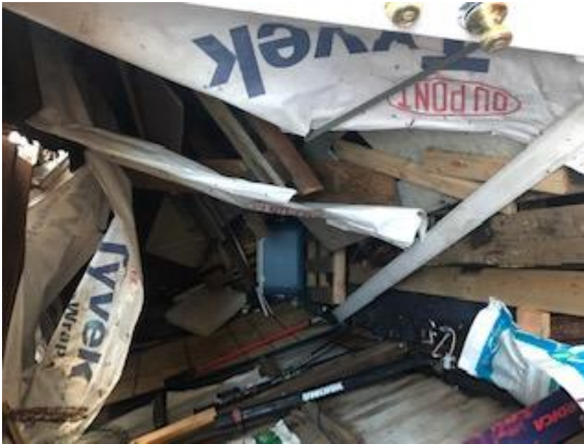
Inside of Garage showing roof collapse
