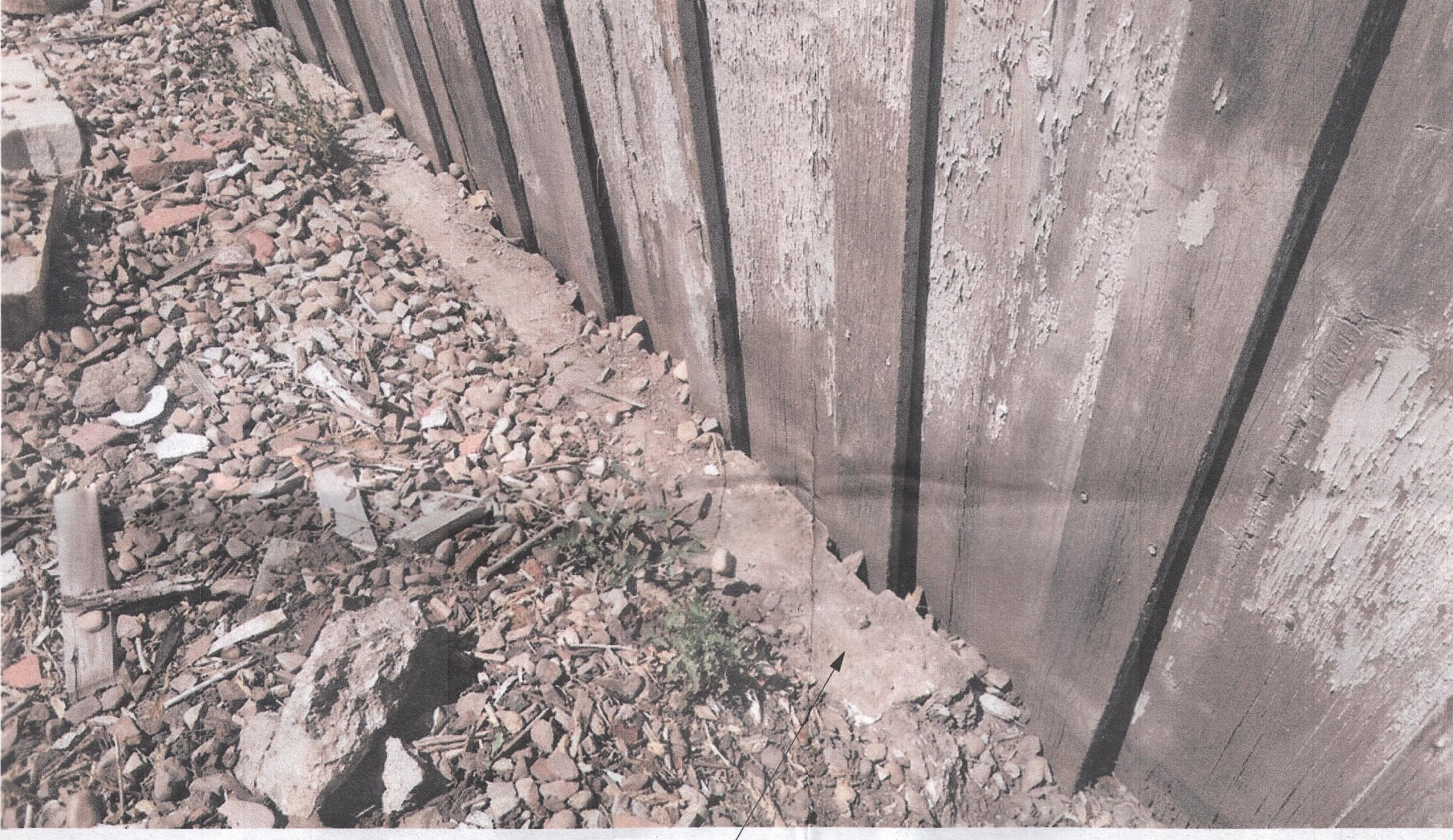
Concrete Poured to Exterior of Shed - Not a Foundation
