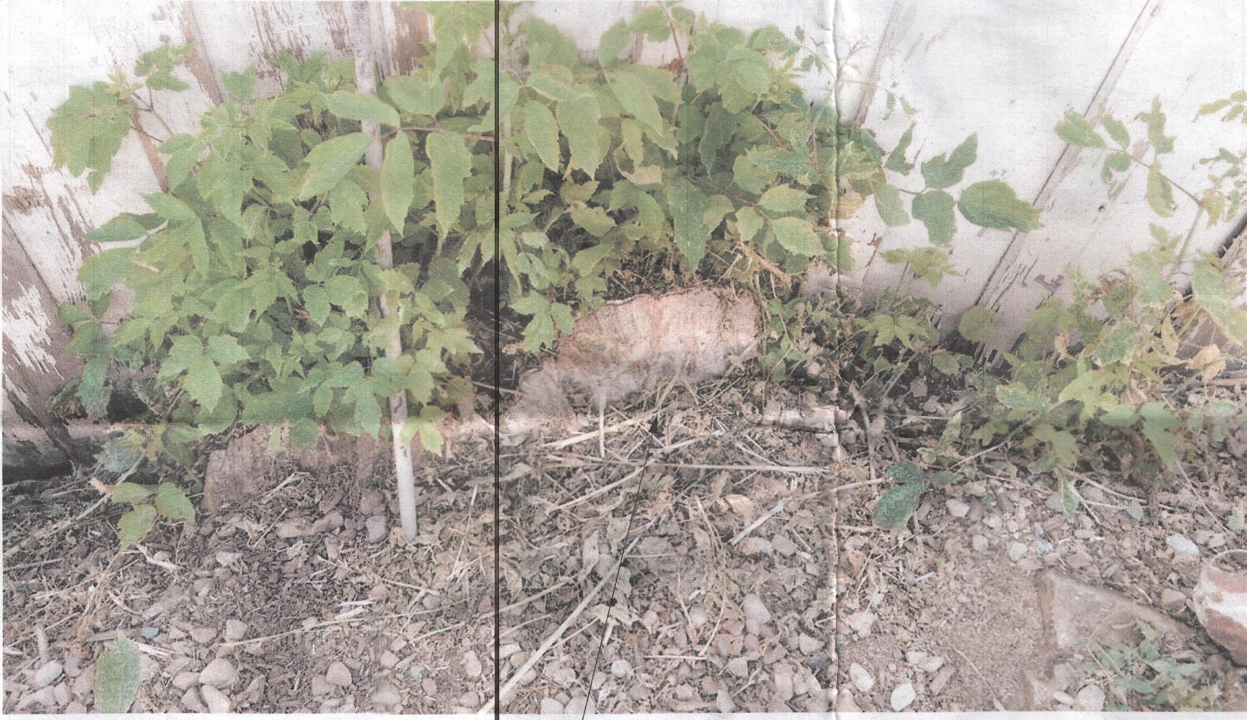
Concrete Poured to Exterior of Shed - Not a Foundation & Pushing Exterior Wall in to Interior of Shed w/ Vehicular Traffic & Pressure on Neighboring Soil
