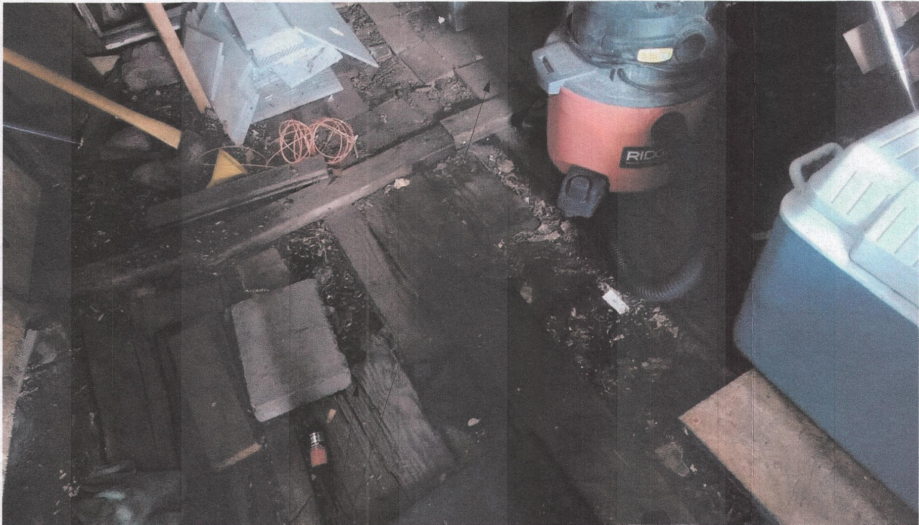
Wood Flooring Directly on Soil - Remove Uneven Brick Directly on Soil - Remove
