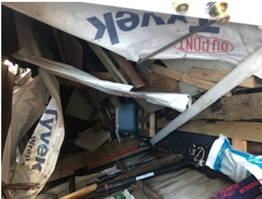
Inside of Garage showing roof collapse
