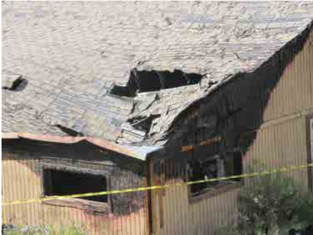
Fire damage at southeast corner
