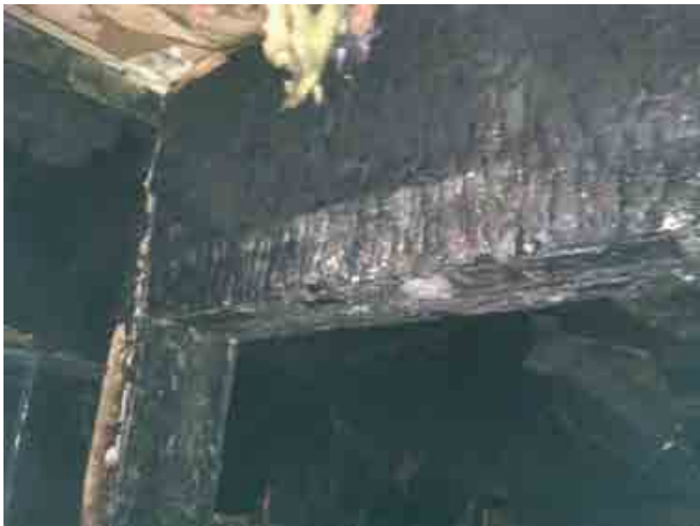
Charred ceiling structure, interior
