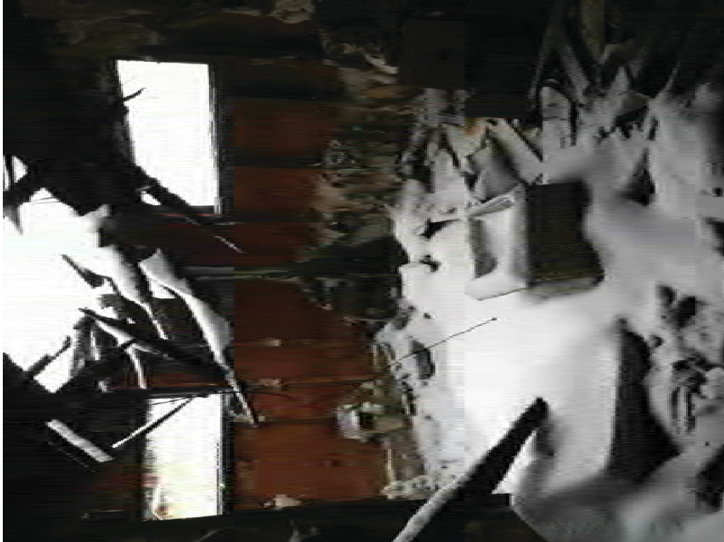
Fire-damaged rear addition. Note the horizontal lumber atop vertical studs.
