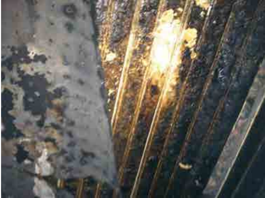
Charred bead-board ceiling in kitchen
