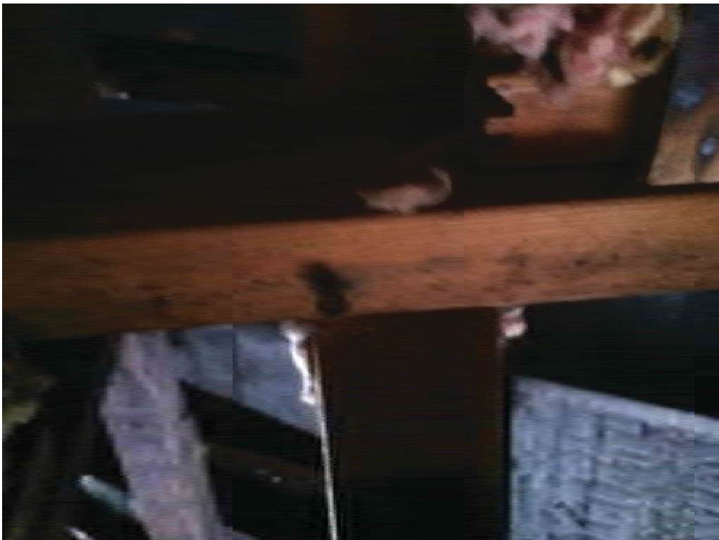
Antique nail and charred roof structure, interior
