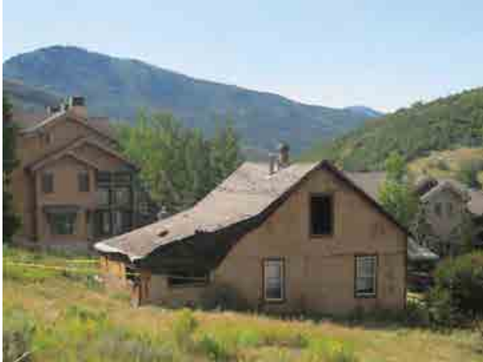
East Elevation (note fire damage)
