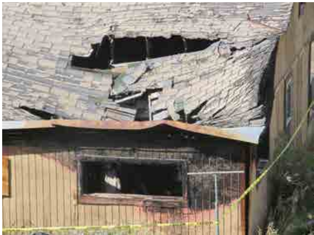
Fire Damage on South Elevation
