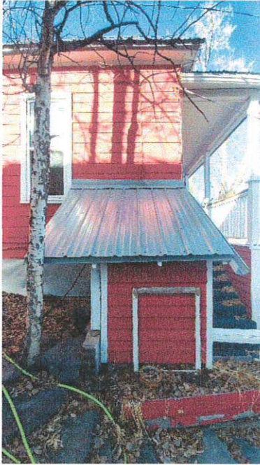
Photo 31: Front Porch Door Non Functioning. (Door E4)
