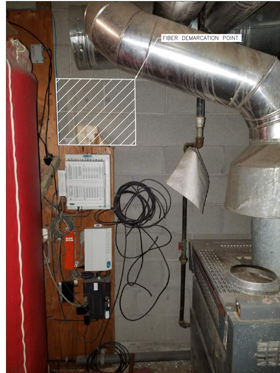
VIEW OF FIBER DEMARCATION POINT
