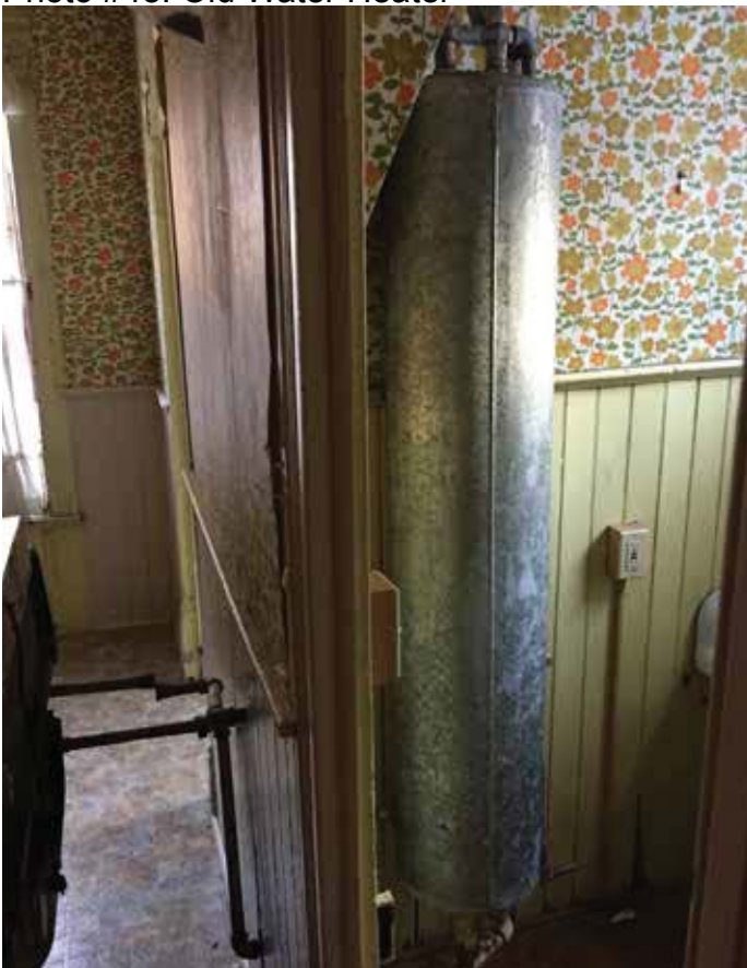
Photo #48: Old Water Heater
