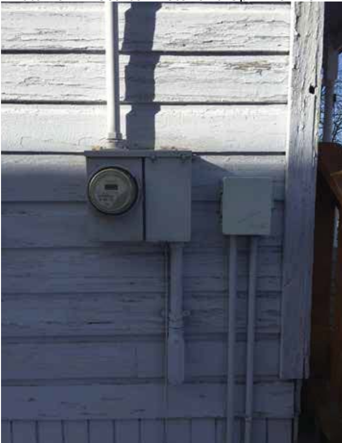
Photo #52: Electrical Meter and Sprinkler Box
