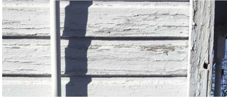
Close-up of siding condition.
