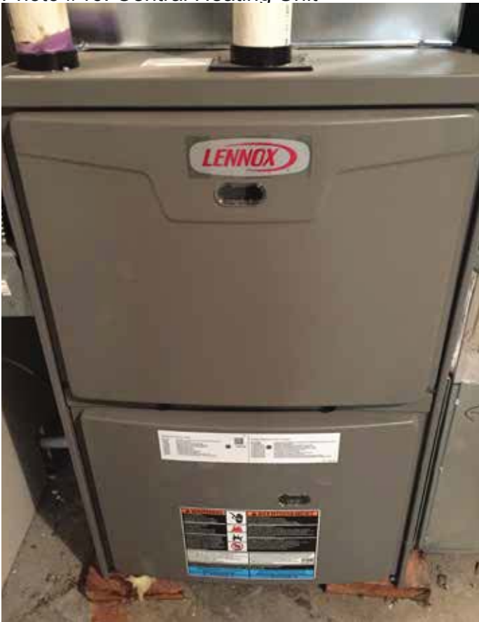
Photo #46: Central Heating Unit
