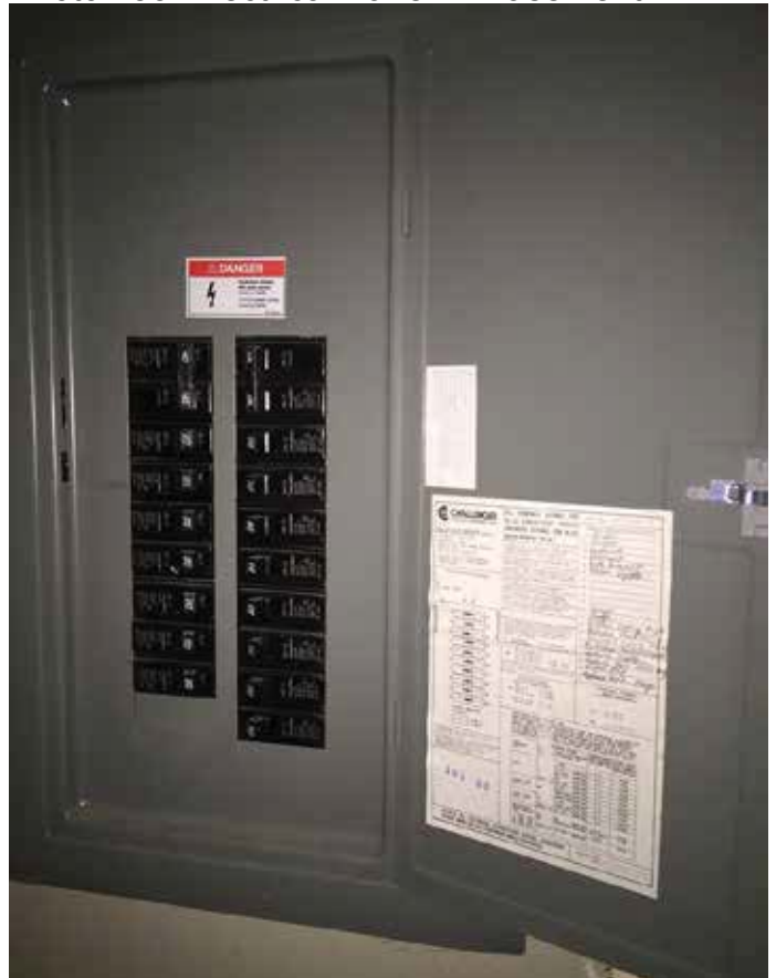
Photo #53: Electrical Panel In Basement
