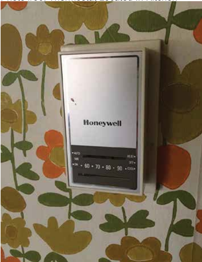
Photo #50: Thermostat Located In Kitchen
