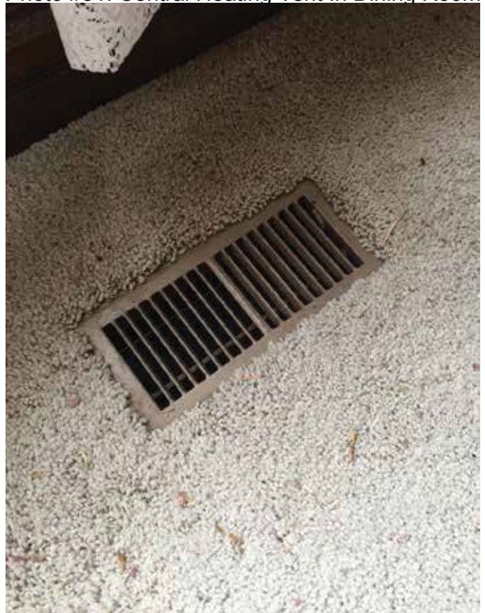
Photo #51: Central Heating Vent In Dining Room
