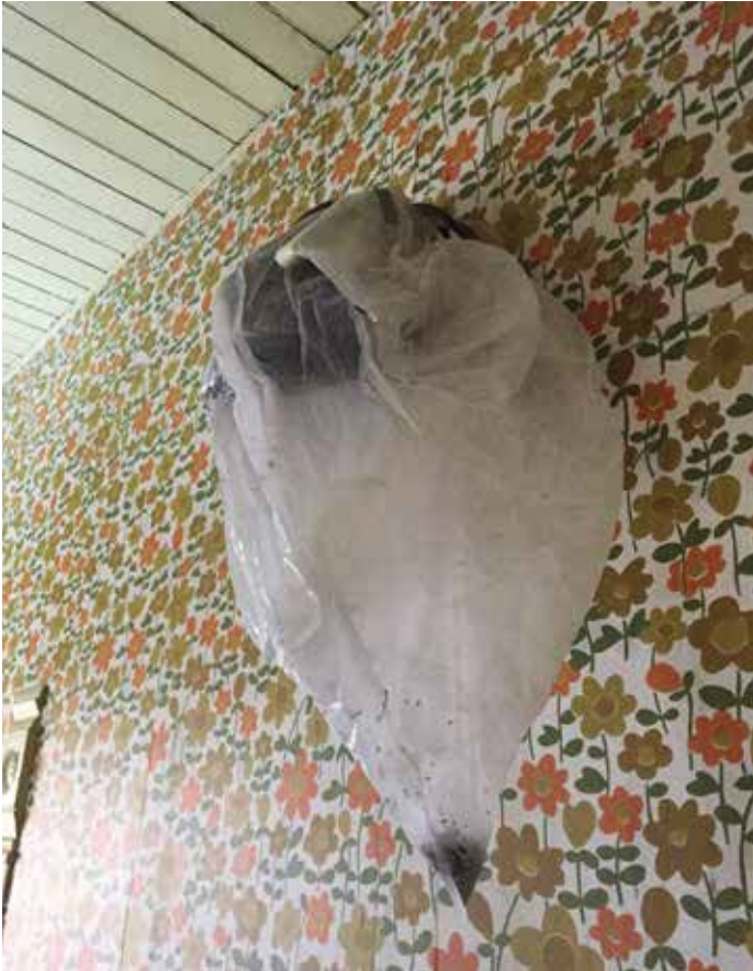
Photo #25: Disconnected Bottom
