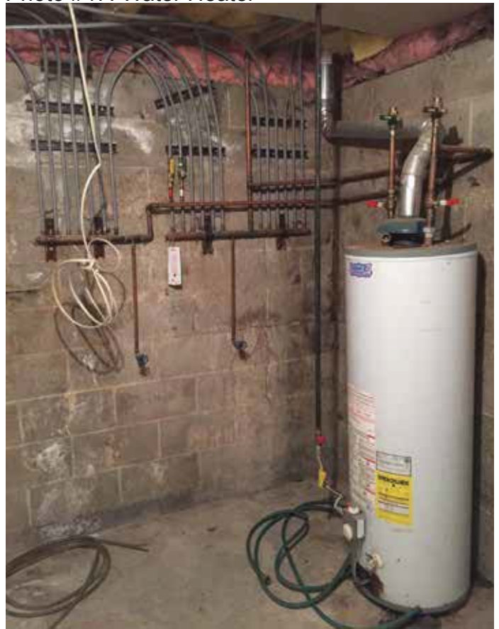
Photo #47: Water Heater
