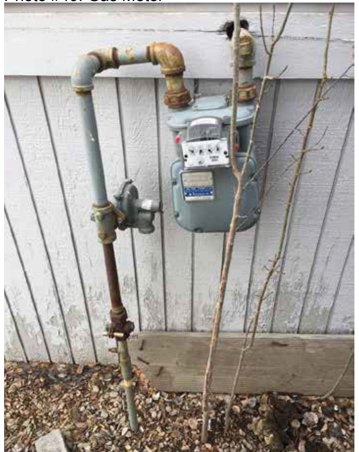
Photo #49: Gas Meter
