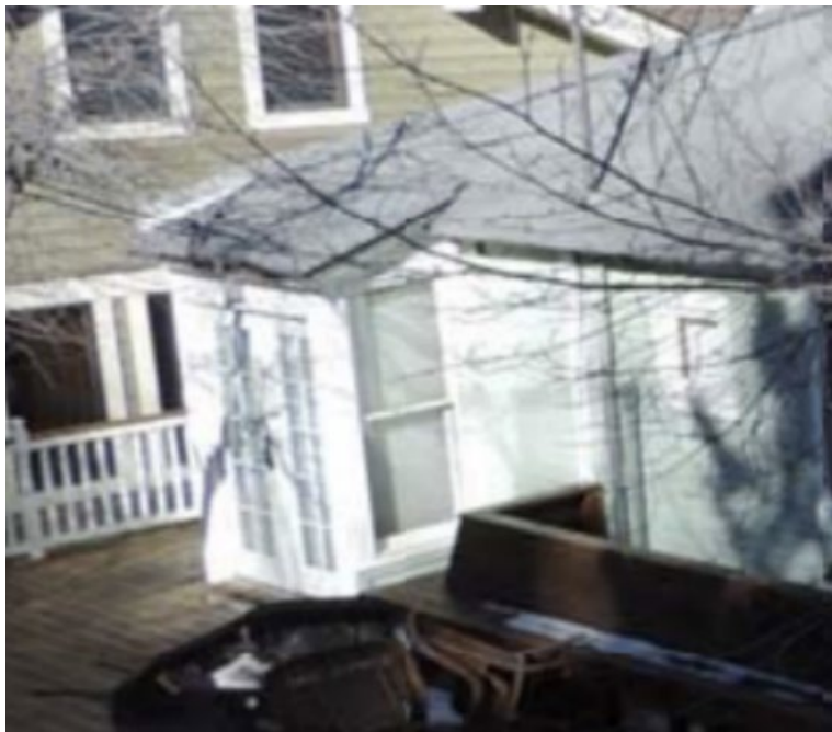
Photo from 2014 (Exhibit E) displaying Existing Bump Out – Altered with the addition of French Doors
