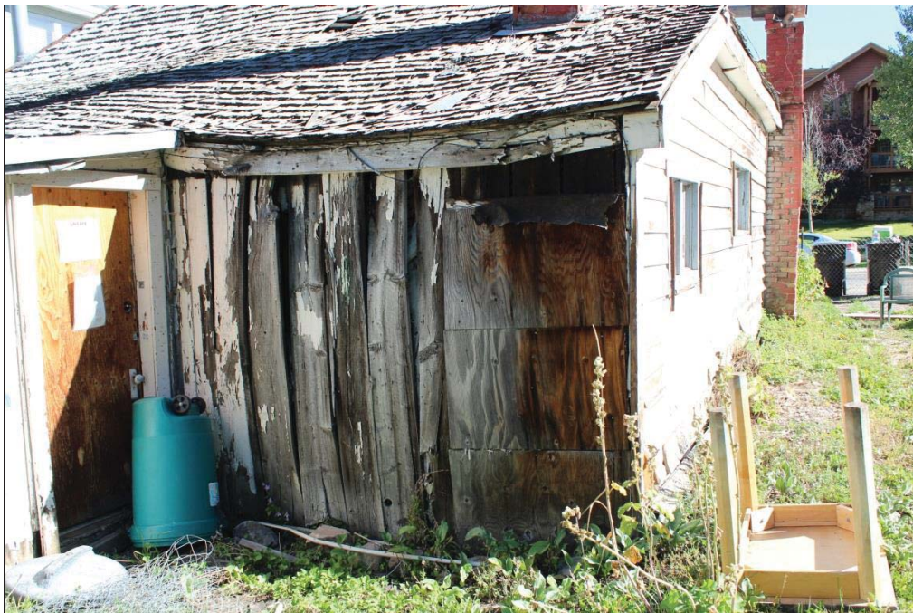
B.4. EXTERIOR WALL – REAR FAÇADE: West side, detail of Addition 1, facing east. Note single-wall construction, very poor condition.
