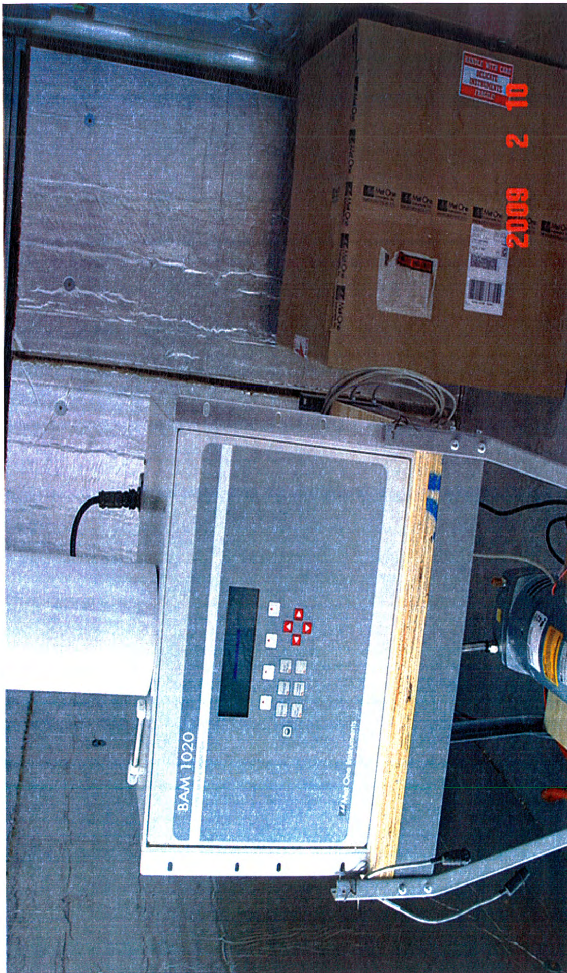
Internal View of Monitoring Station
