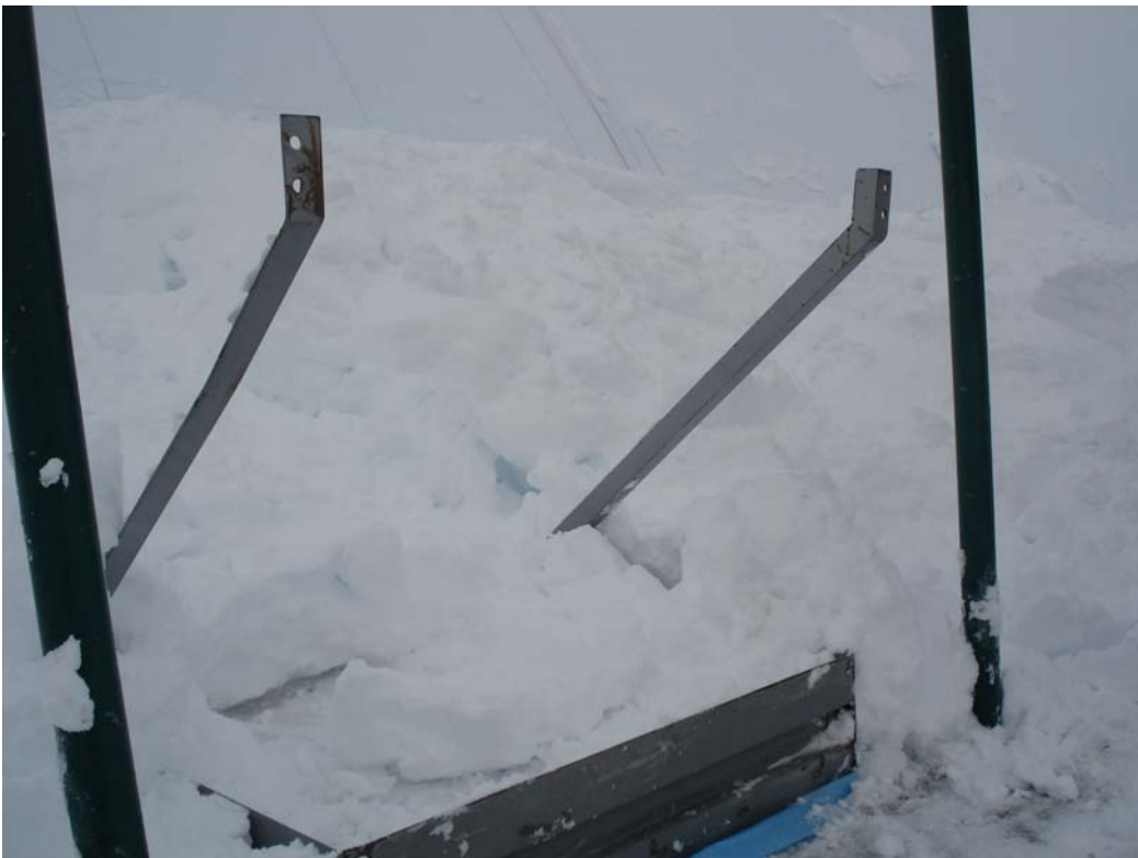
The snow load caved in the emergency door.
