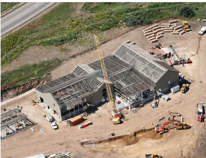
Quinn's Junction Water Treatment Plant, July 2011
