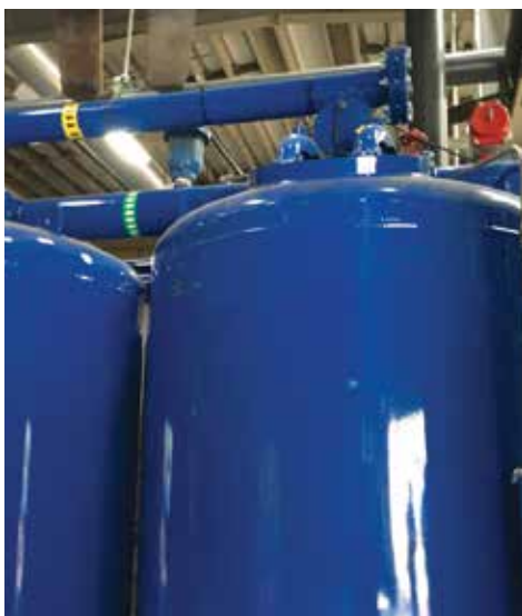
Quinns Junction WTP manganese filters
