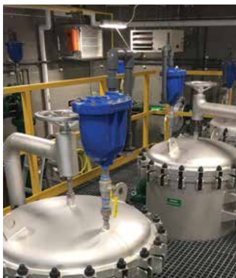
Creekside WTP filters
