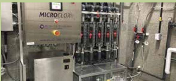
On-site chlorine generation
