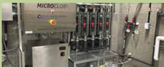
On-site chlorine generation
