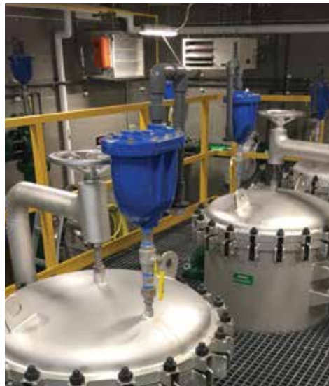
Creekside Water Treatment Plant filters
