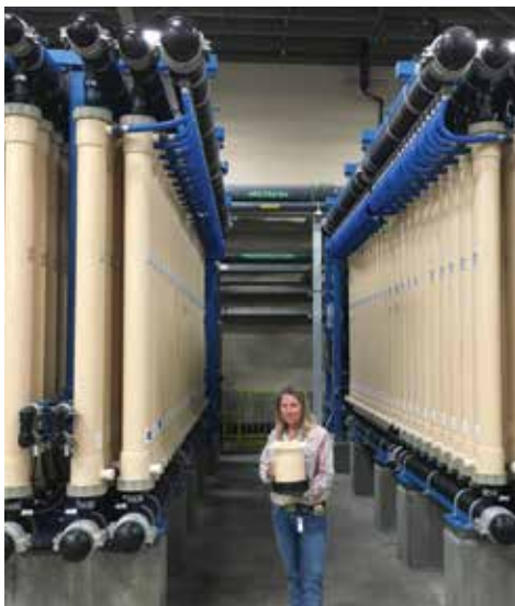
Quinns Junction Water Treatment Plant microfilters
