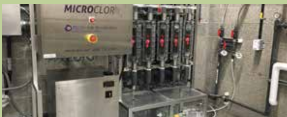
On-site chlorine generation
