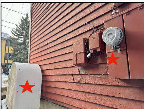
Shows the water meter and electrical meter at 948
