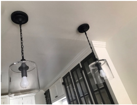
Figure 9: Dry Wall Sagging
