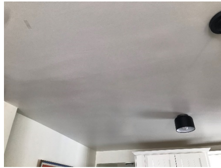
Figure 10: Dry Wall Sagging
