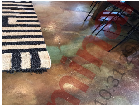
Figure 20: Cracking In Bottom Floor Slab
