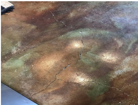
Figure 19: Cracking In Bottom Floor Slab
