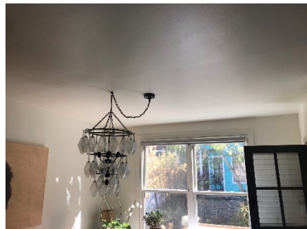
Figure 8: Dry Wall Sagging
