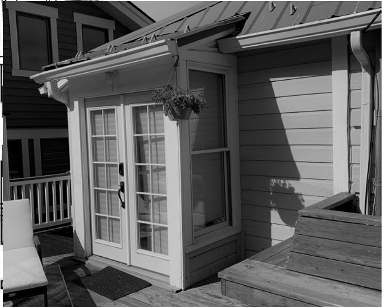
Current bay w/ Windows replaced by non-historic doors
