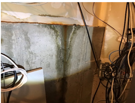
Figure 21: Wet Foundation Wall
