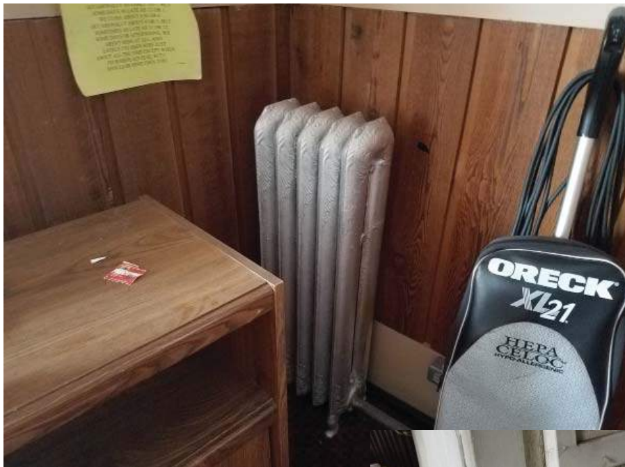
77 - L1 - Dining Room Radiator
