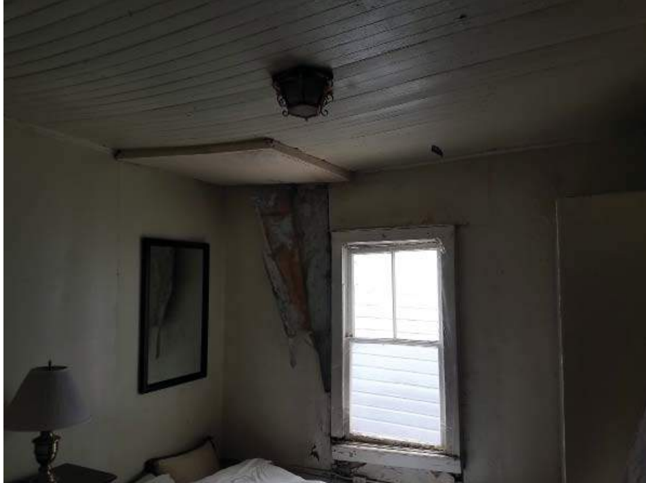
92 - L2 - Sagging Ceiling in Bedroom 207
