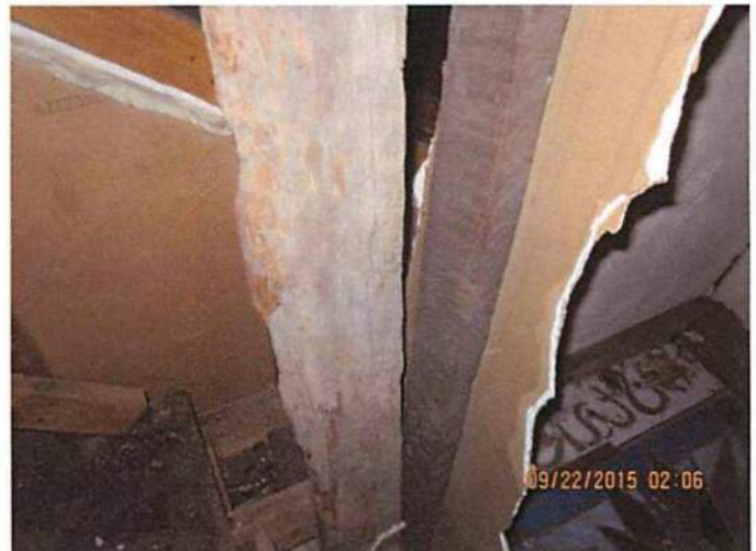
Photo 4 Structural members not properly supported
