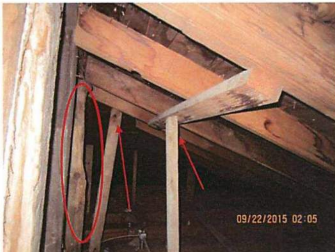
Photo 3 Damaged, decayed or improperly installed structural members
