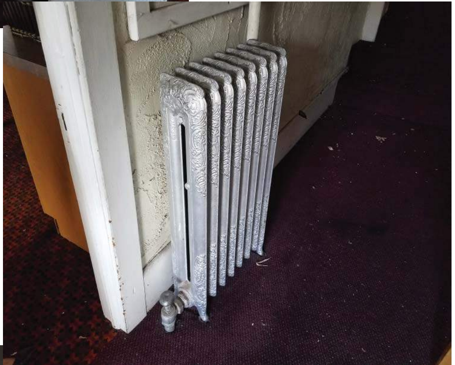
78 - L1 - Typical Radiator
