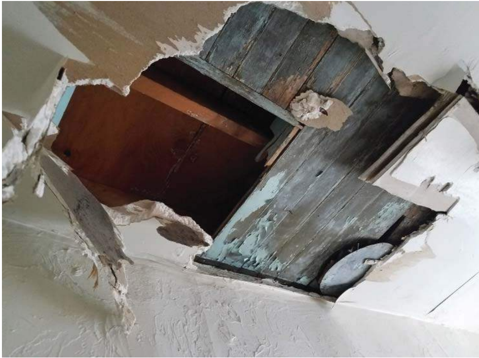
91 - L2 - Sagging Ceiling in Bedroom 206
