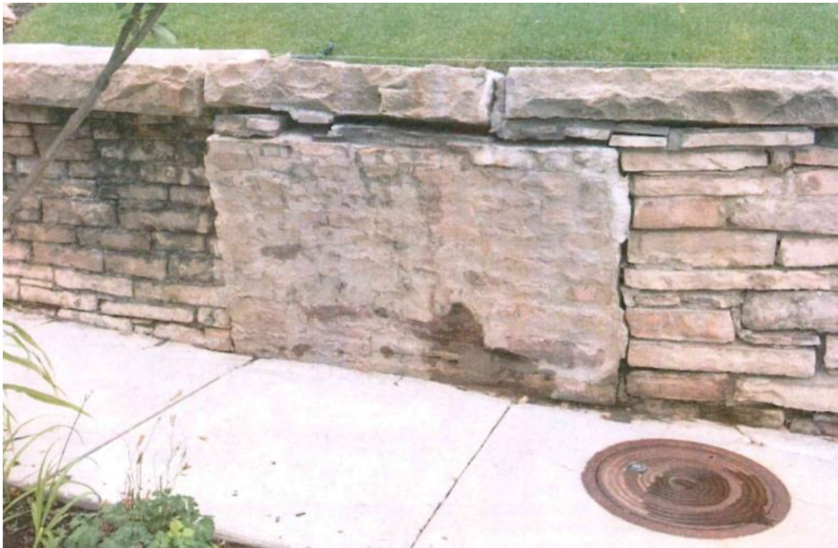
Figure 3: Historic wall in 2018 prior to repair.
