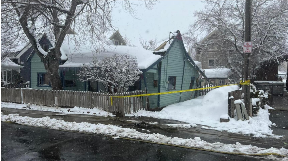
Park Ave. home roof collapse Photo: PCFD
