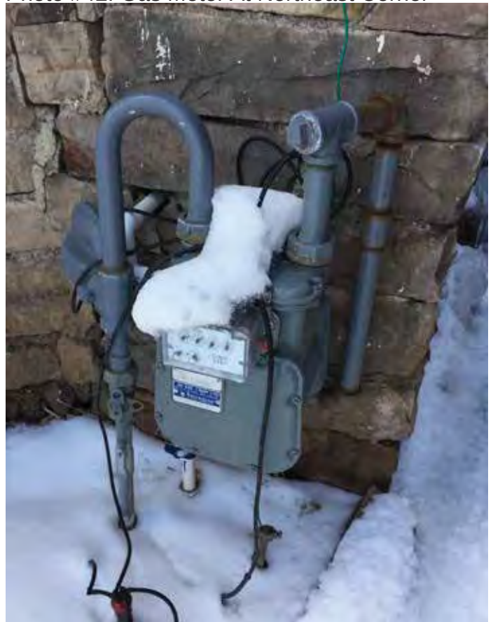
Photo #42: Gas Meter At Northeast Corner
