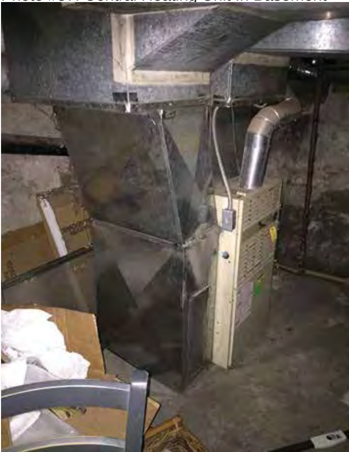
Photo #37: Central Heating Unit In Basement
