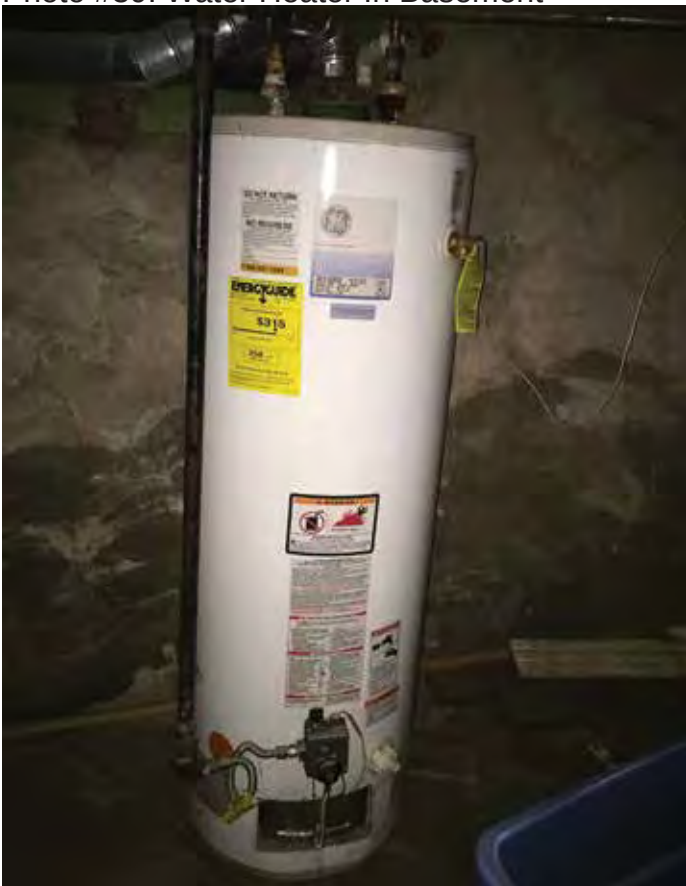
Photo #39: Water Heater In Basement
