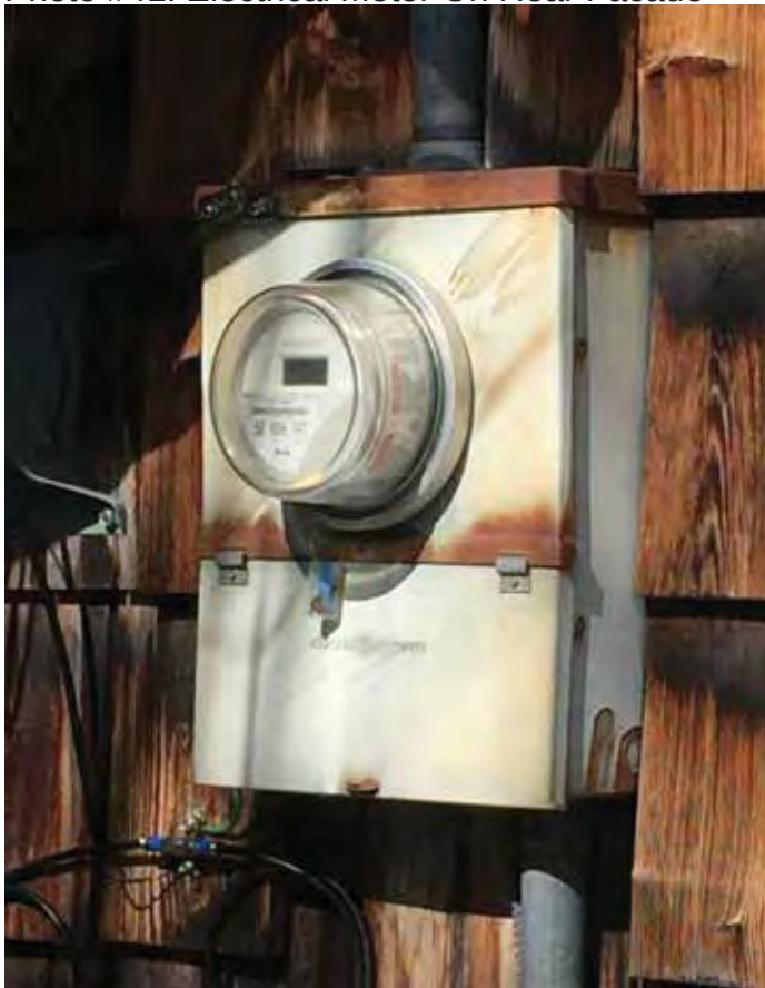
Photo #41: Electrical Meter On Rear Facade
