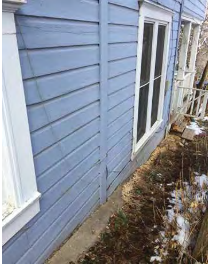
Photo #33: Exposed Foundation At South Facade
