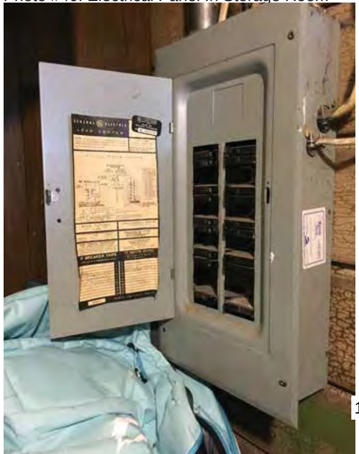
Photo #40: Electrical Panel In Storage Room
