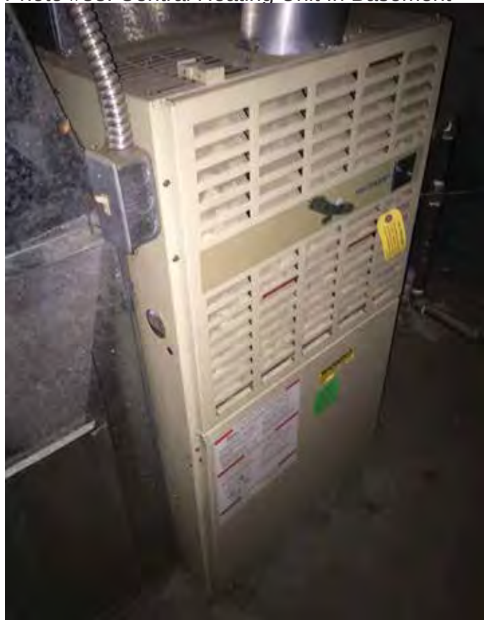
Photo #38: Central Heating Unit In Basement
