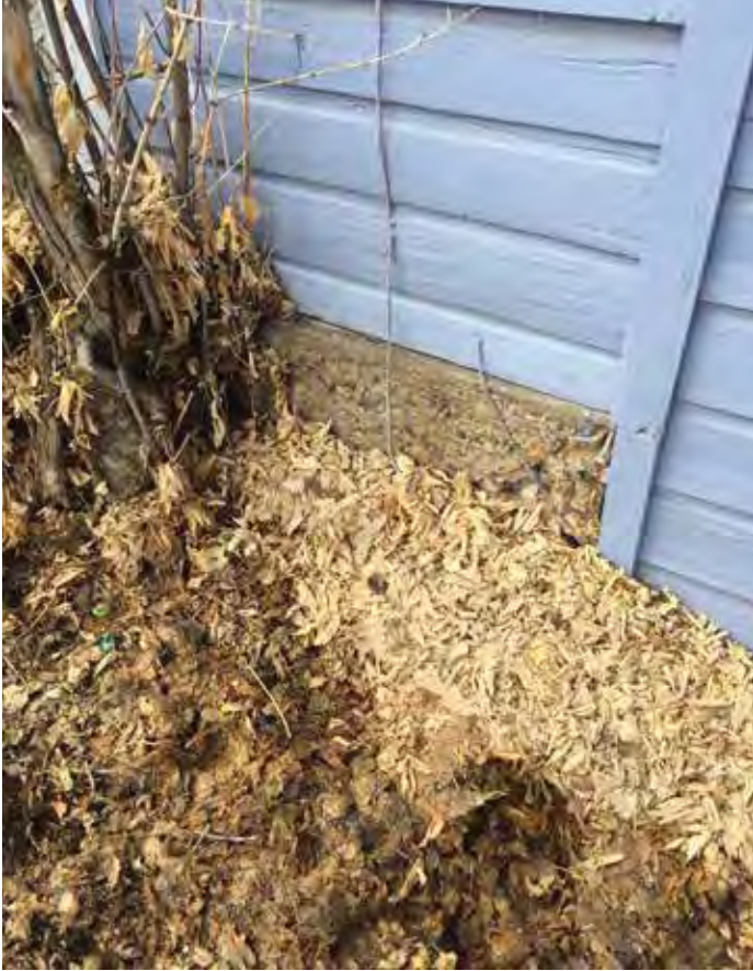
Photo #32: Exposed Foundation At Rear Corner
