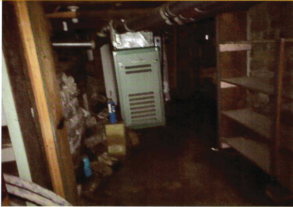
Photo 1: Excavated Basement with Collapsed Brick
