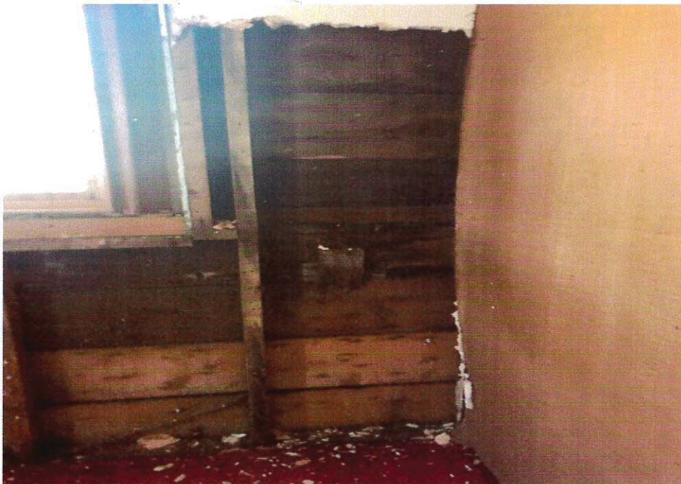
Photo 4: Sagging Floor Corner and Historical Studs/Slats
