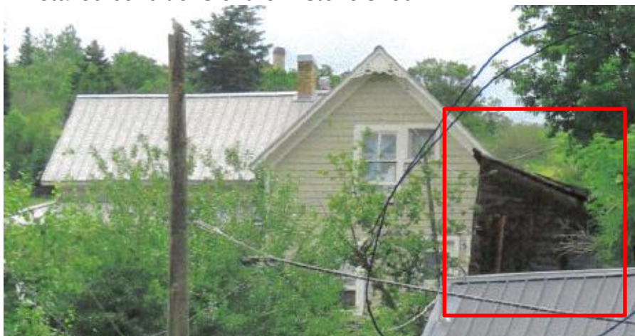
Figure 2: Detailed conditions of the Historic shed.
