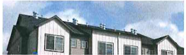
Mechanical vents reflect architectural style
