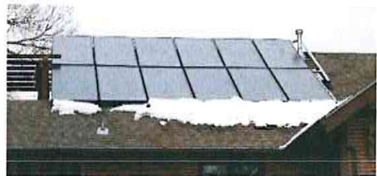
Solar panels visual impacts are minimized
