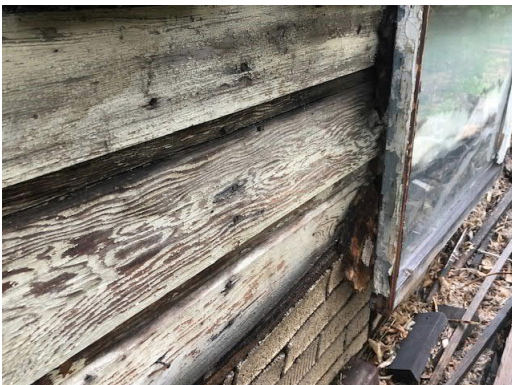
Photo #7 Lead-containing paint on the west side of the south shed.
