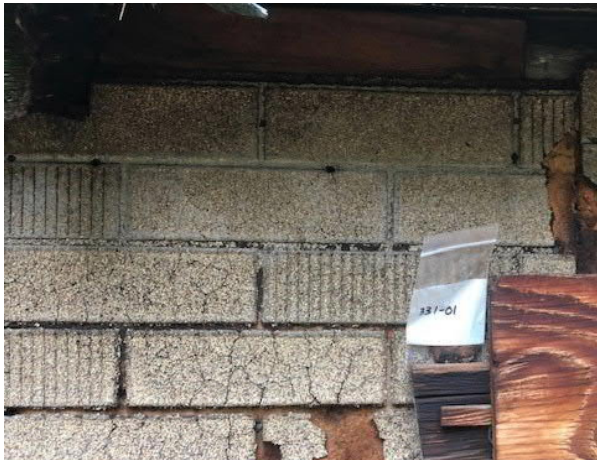
Photo #1 Sample 331-01. Tan brick pattern tar paper with wood fiber backing; south shed – not asbestos containing.
