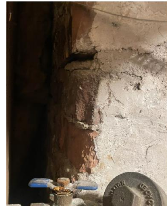
Figure 7: Damaged chimney mortar
