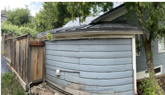
Figure 5: View of southern facade, showing water damaged siding
