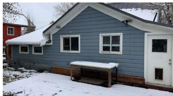
Figure 6: View of western (rear) facade, showing water damaged siding at northern end
